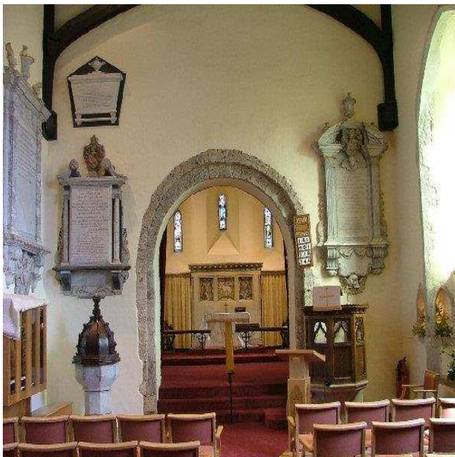
Figure 61: Monumental tufa arch showing heavy weathering on the original external and internal faces, All Saints Church, West Farleigh. Likely re-used from the East Farleigh villa site. Simon Elliott.
