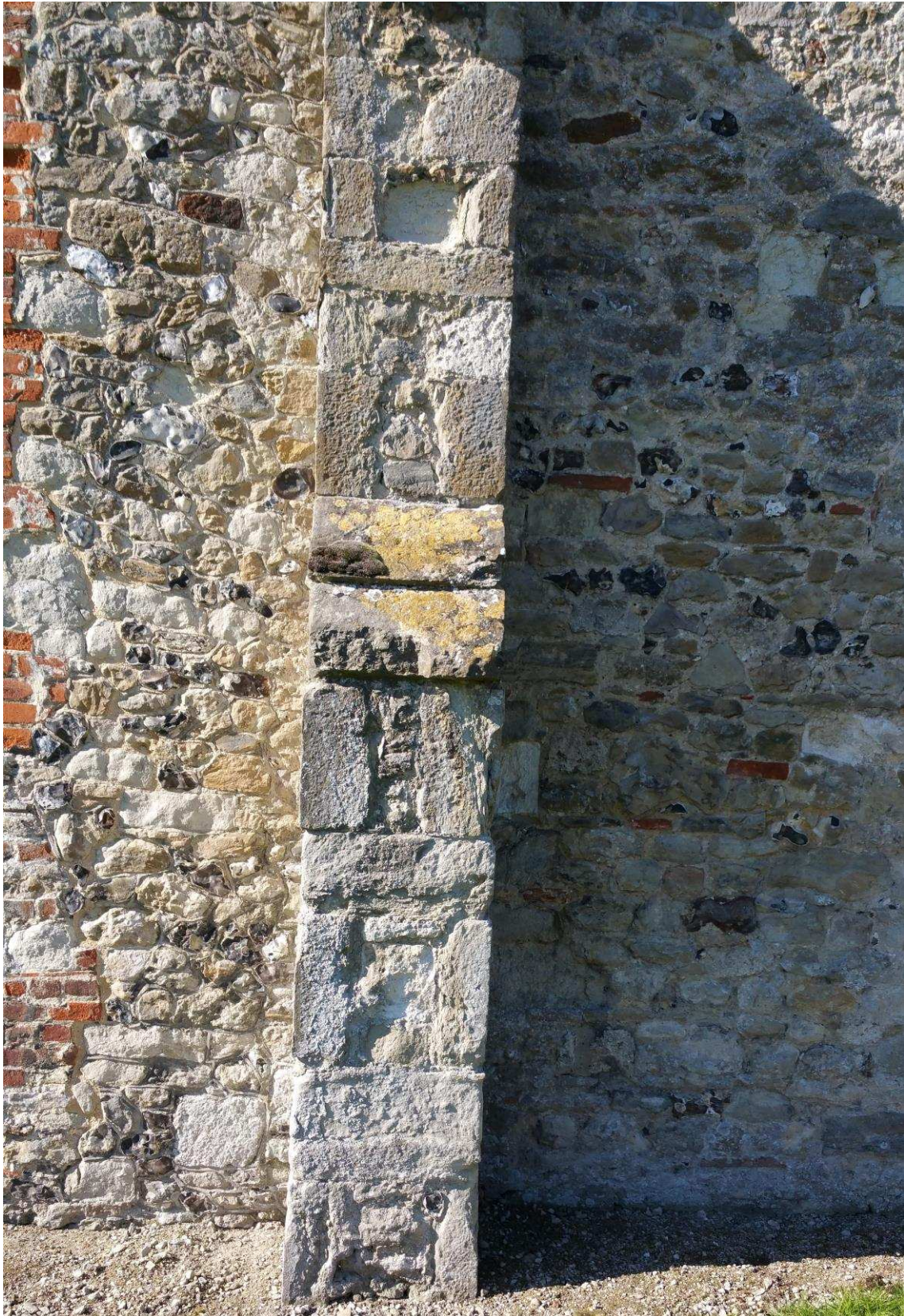
Figure 48: Ragstone, chalk and tufa blocks from the Roman villas at Court Road and Eccles re-used in buttresses of St Mary's Church, Burham. Simon Elliott.
