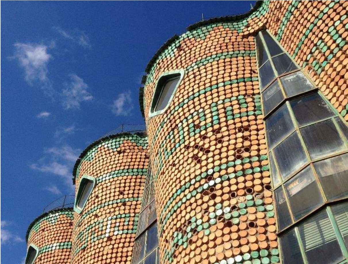
Figure 15. Solimene Ceramic Factory, Vietri sul Mare, Salerno, 1956, Architect Paolo Soleri. The present state of the façade with the several vases damaged over the time (January 2016). (Photo: Luciano Cardellicchio)
