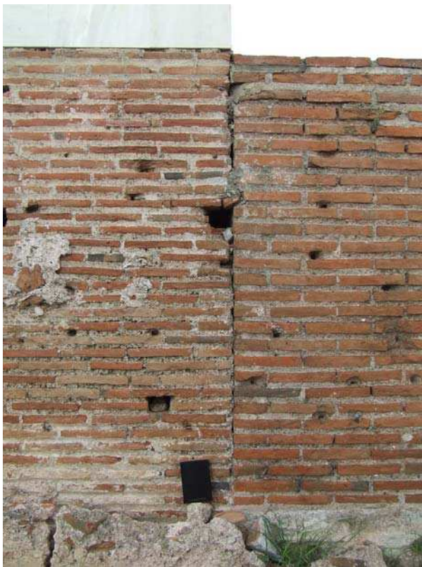
Figure 13. Detail of the vertical joint between the external walls of the nave and the transept.
