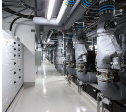
Plant space in 20 Fenchurch Street
