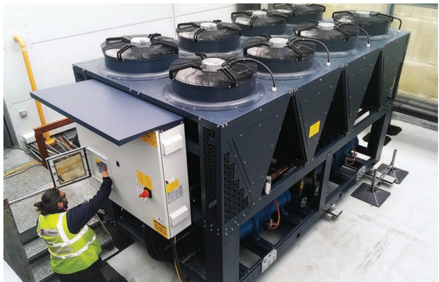
Figure 1: A 500kW air-cooled propane chiller (Source: Cool-Therm)
