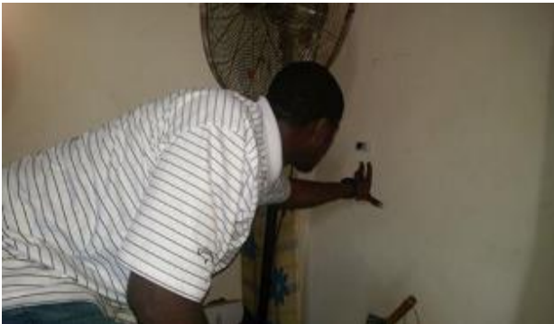
Fig 4: Installation of HOBO Temp/Rh indoor loggers
