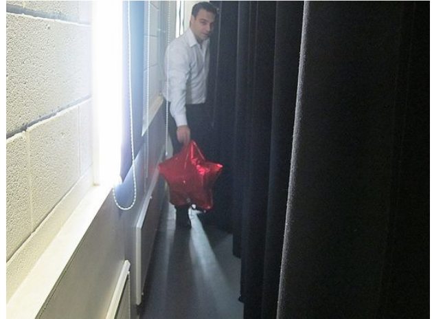
Fig 4: Testing behind the curtains, and showing the perimeter Passivent air inlet grilles
