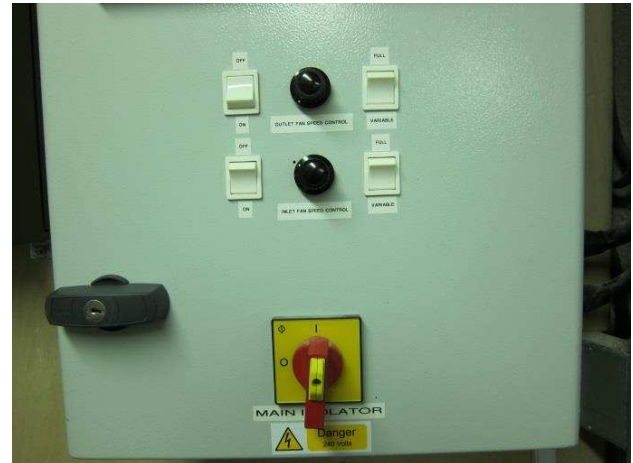
Fig 7: Fan control panel
