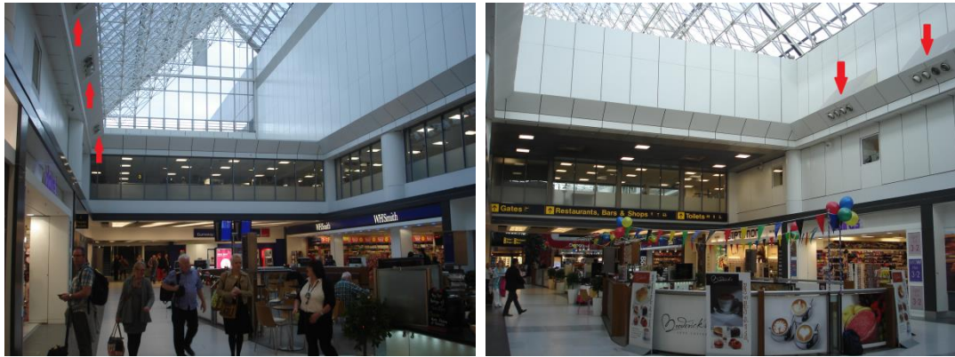
Figure 6-60: Air-conditioning nozzles positioned immediately beneath the roof in the seating area, MAN T2.
