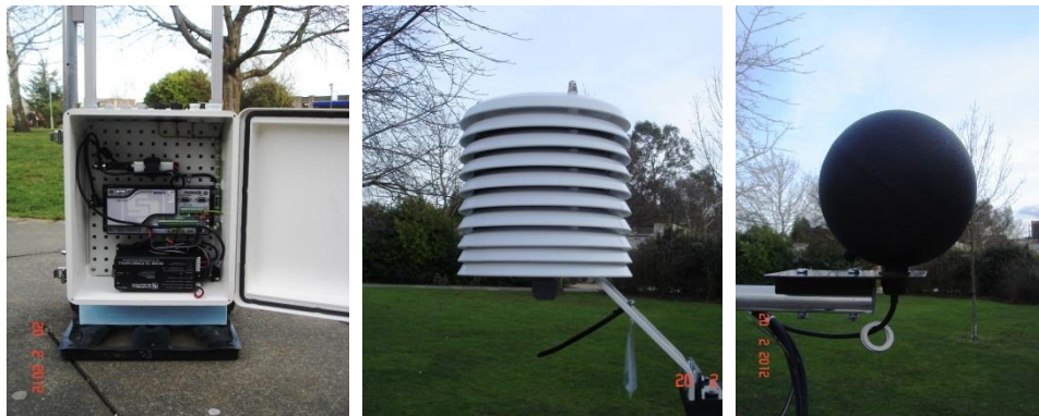
Data logging system & battery
