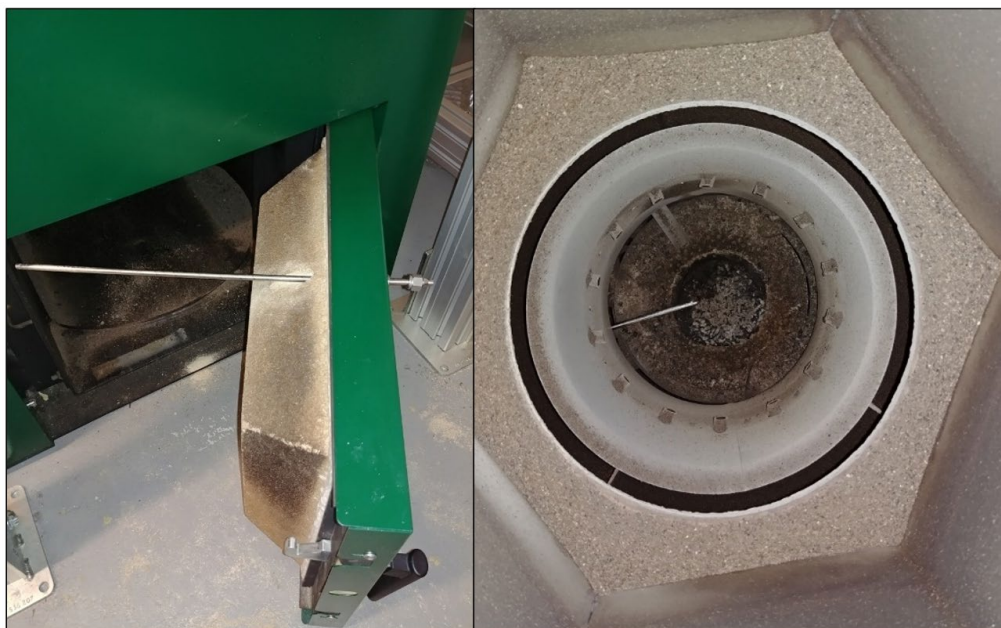
Figure 3-8 Passage of the probe through the door wall and its positioning in the flame
