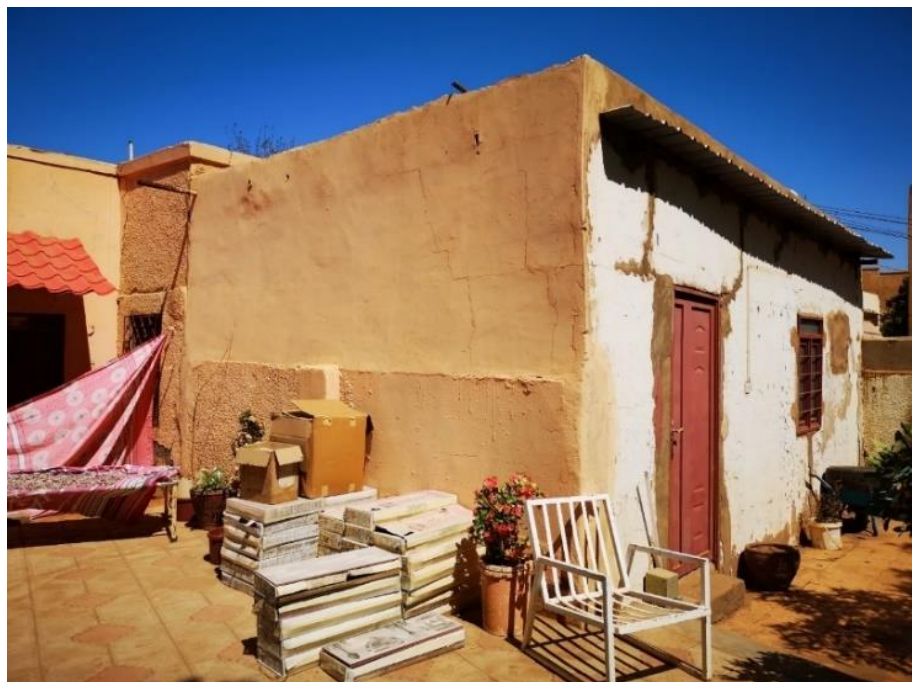
Figure 5.16 A photo of T1 showing the haphazard extension built over the boundary wall
