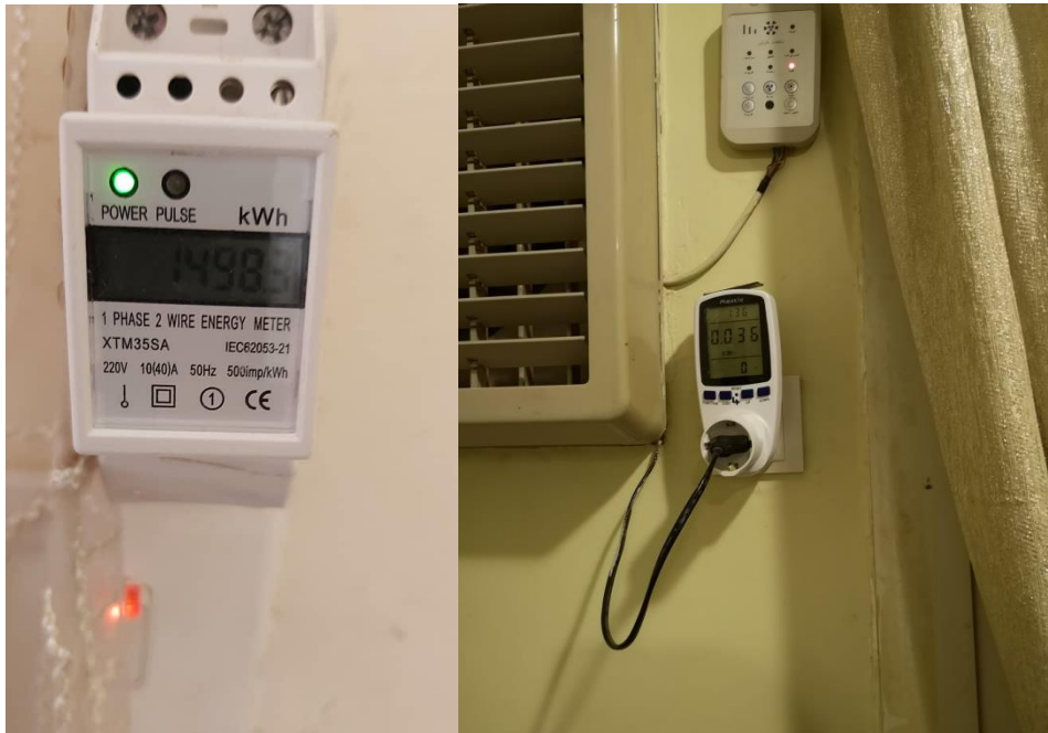
Figure 3.5 Left: shows the meters installed at the split unit in M1. Right: the plug in meters used for the evaporative coolers
