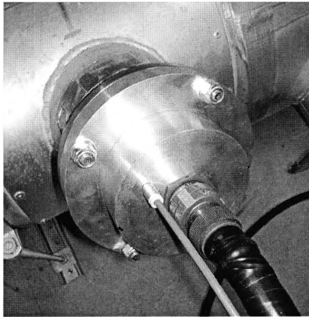
Figure 5.32: Optical/electrostatic integrated sensor installed on pipeline
