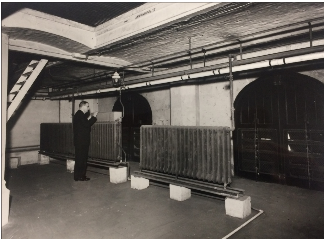
Figure 10: Interior of the air chamber, 4 March 1966, showing the adjustable louvres of the intakes.
