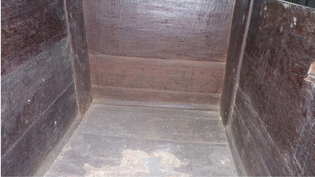
Fig 13. Internal view showing smooth surfaces with quarter-round lip, St John's A . Photograph: author.
