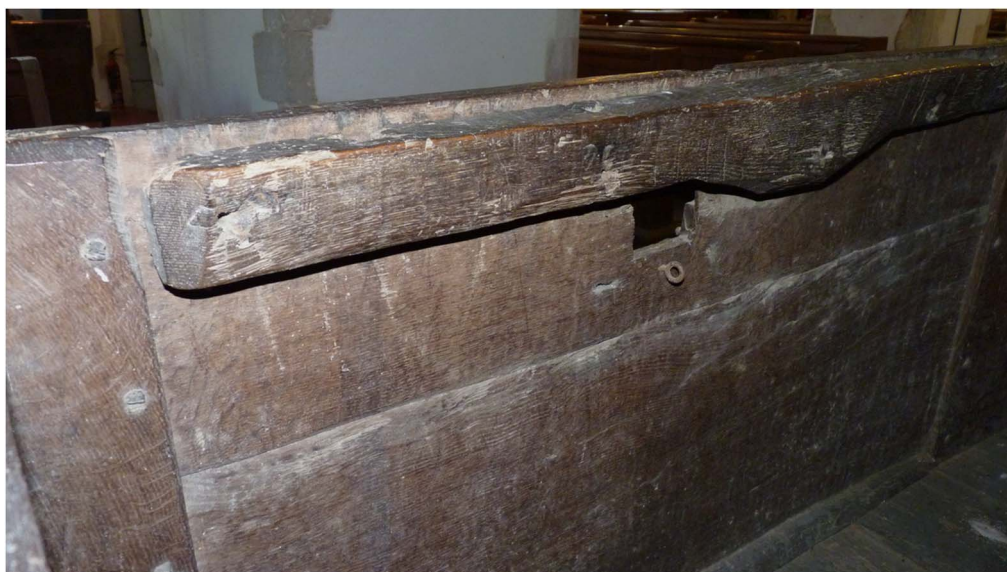
Fig 16. Wooden sliding bolt cover, quarter-round lip above bottom boards, Wormshill. Photograph: author.
