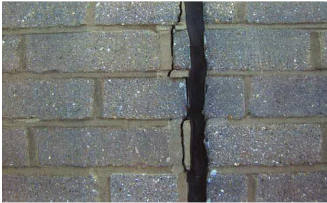
Figure 4.4. Close up of cracked brickwork and spalling joint filler (ECD Architects, 2015).
