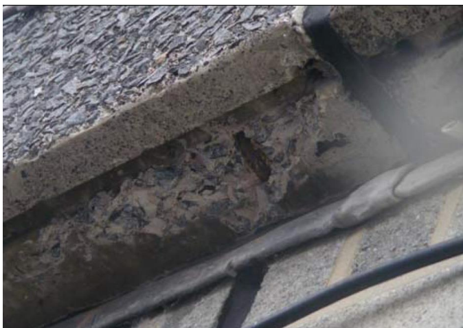
Figure 4.5. Spalling at base of panel in [REDACTED] (ECD Architects, 2015).
