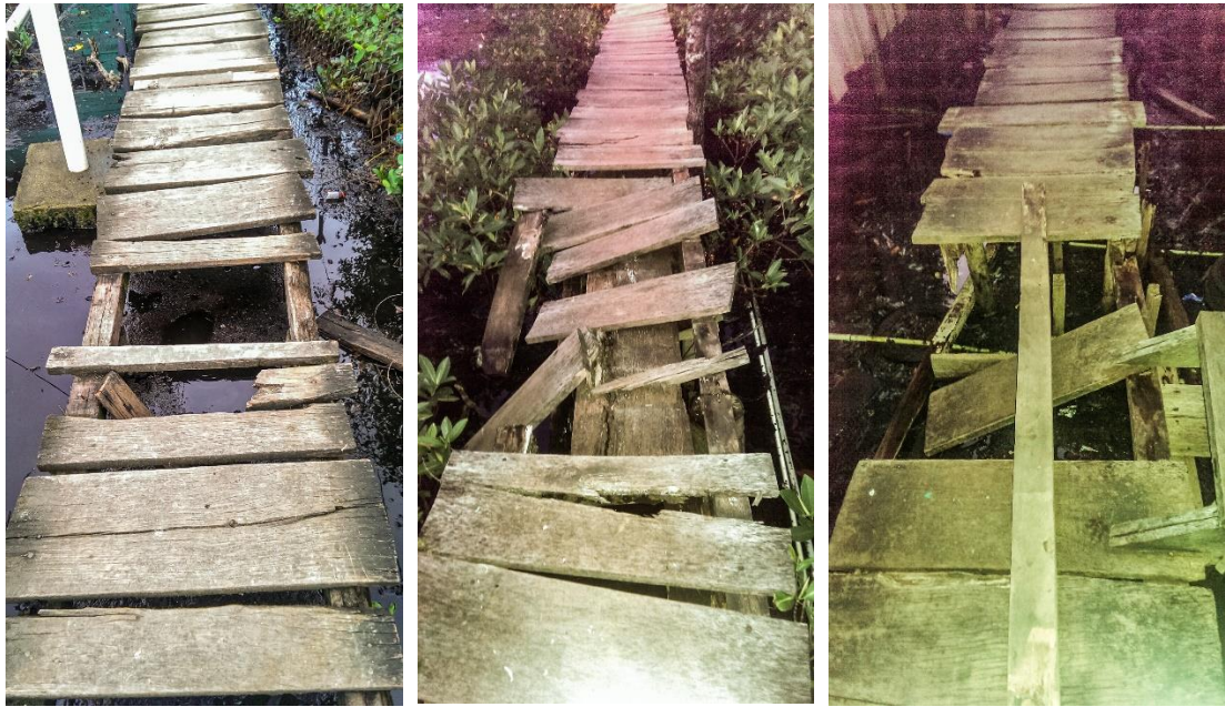
Figure 22: Muelle - boardwalk (in disrepair)
