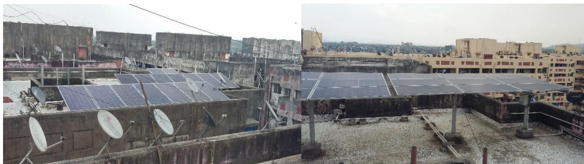
Figure 2: Solar panels installed on the rooftop of the buildings in Natwar Parekh Colony (photograph taken by Anika Haque, 2018)
