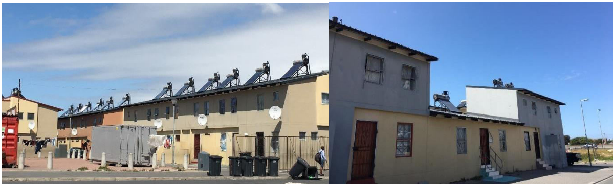
Figure 4: Solar water heaters installed on housing units as part of the Joe Slovo SWH project (photograph taken by Sayd Kusai, 2019)
