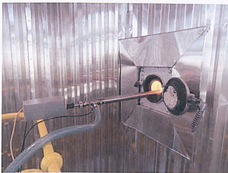
Figure 6.5 Flame imaging system and its installation
