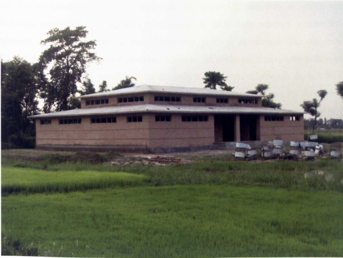
Figure 7.2: The recently completed Tharu Culture Museum, built to mimic the architecture of the traditional Tharu house, and awaiting internal fittings
