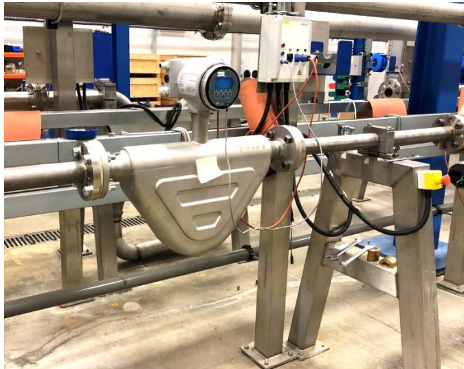
Figure 5.13 Photo of the Coriolis flowmeter under test (CF2) with belly down
