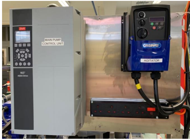
Figure 3.4 Motor control panel of centrifugal pump and agitator
