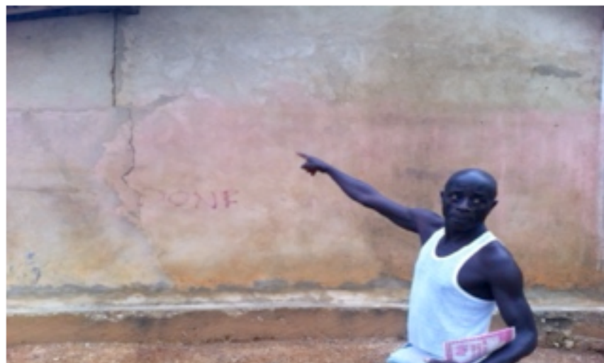
5.7: A Dumasi Community resident pointing out the damaging cracks to one of many houses as a result of the frequent dynamite blasting by the mining company. No compensation or cost of repair has been paid. Source: Author's own (picture used with permission).
