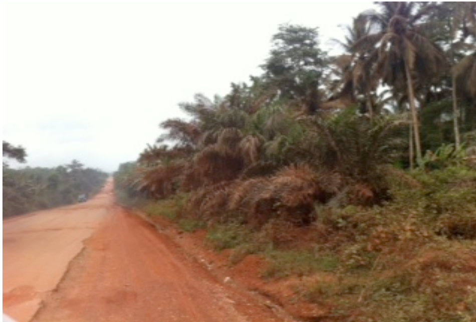
Main road leading to the Dumasi very poorly constructed (half surface tar eaten away) and dusty. Note the Palm fronds and vegetation looking very brown from settled red dusty.
