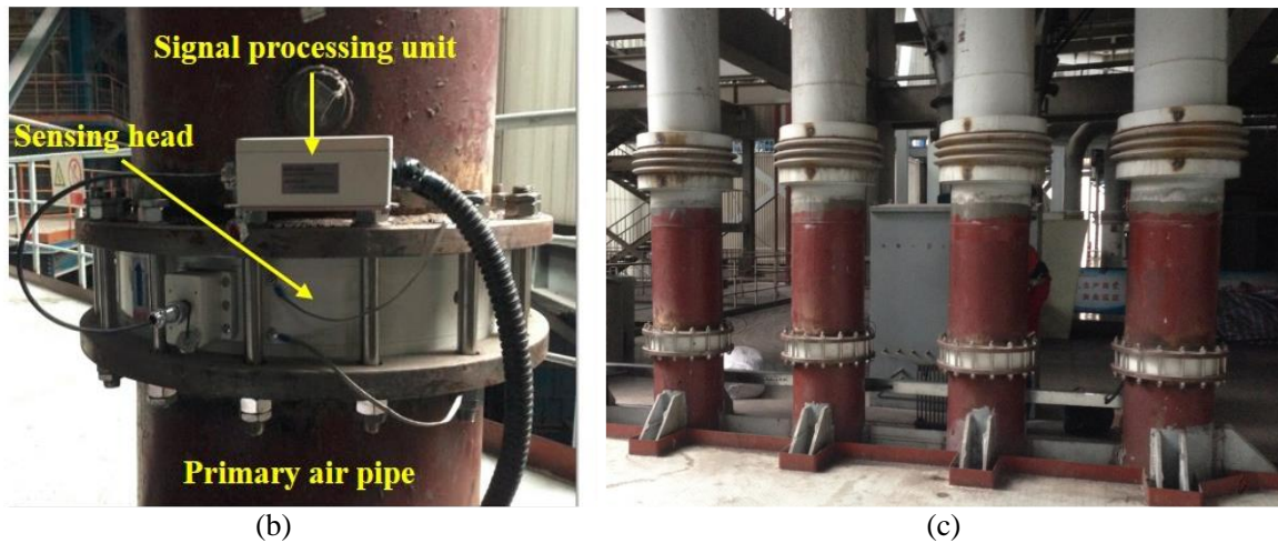
Fig. 10. Application of the PF flow measurement system with five electrostatic sensing-heads. (a) Schematic of the measurement system on a furnace. (b) Installation of the electrostatic sensing head. (c) A set of four sensing heads on the same pulverising mill [27]. Copyright © 2017, IEEE
