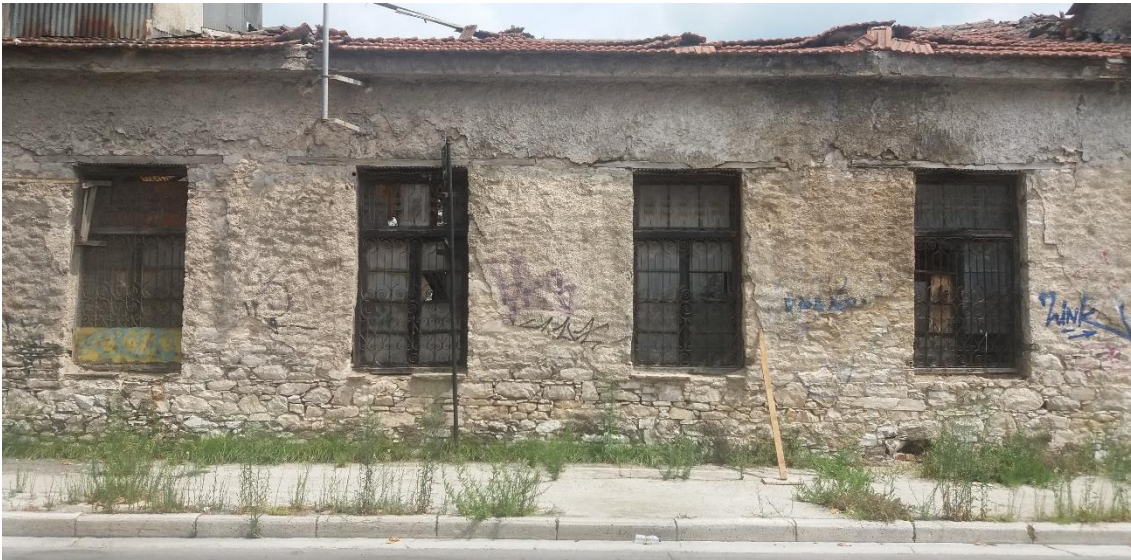
Fig. 12. The Machine Shop, view from Papdiamantis Street. Note the load bearing structure of the Machine Shop which belongs to one of the earliest surviving assets on site.
