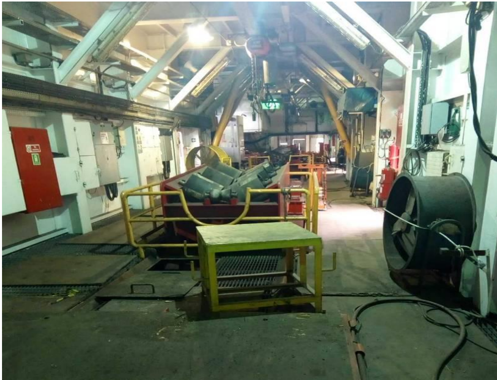
Figure 2: A typical engine room of a barge operating in WA
