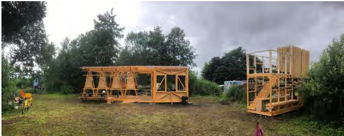
Figure 1: Test Unit, showing main pavilion (left) and 'The Nettle Inn' (right) under construction.
