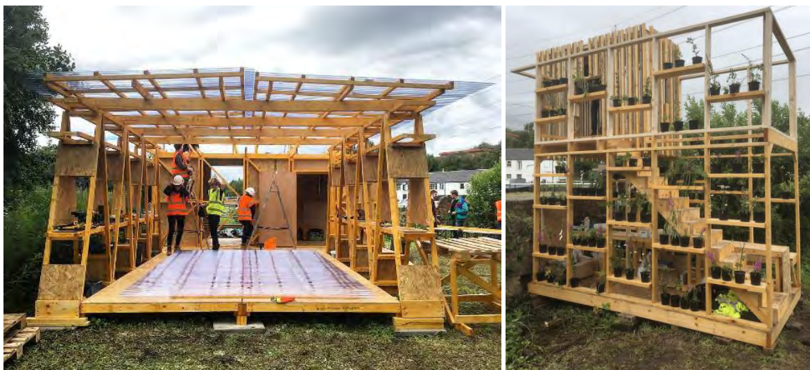
Figure 2: Test Unit, showing main pavilion under construction (left) and 'The Nettle Inn' (right).
