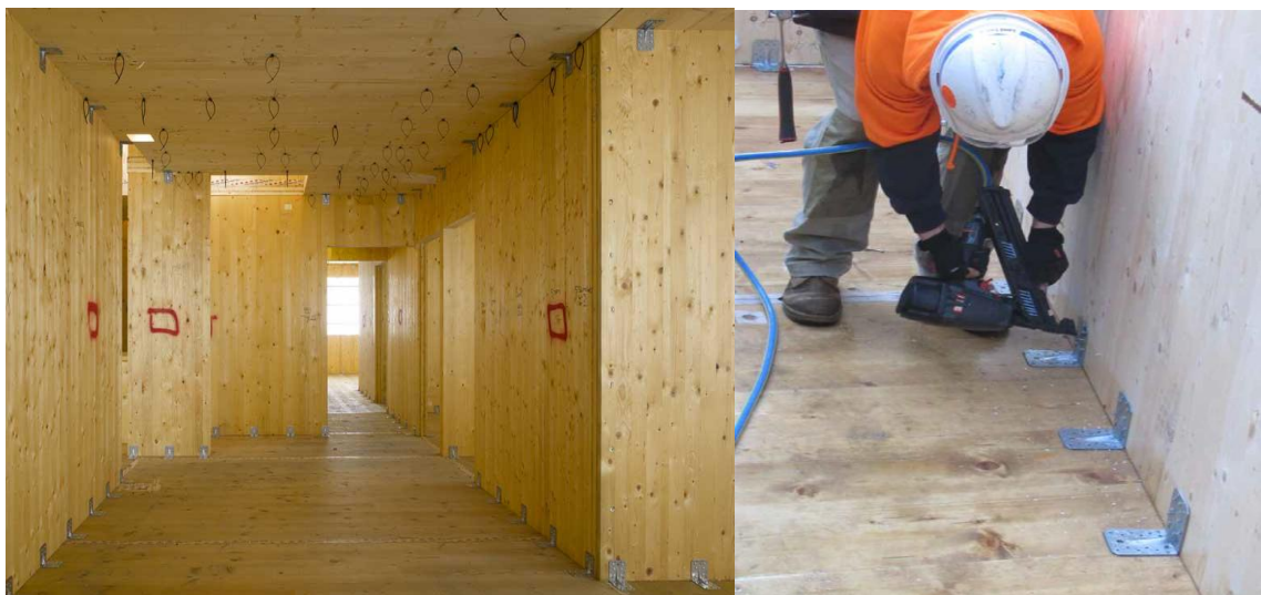
Figure 5.23: The interior of Stadthaus showing the connection between wall and floor timber panels (left) (Thompson, 2009); using angle platters and screws for connection (right) (Wood Solutions, 2013).
