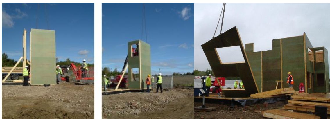
Figure 5.18: Arrangement of the panels using light equipment on the concrete ground floor constructed over strip foundation at Oxley Woods (RSHP Architects).
