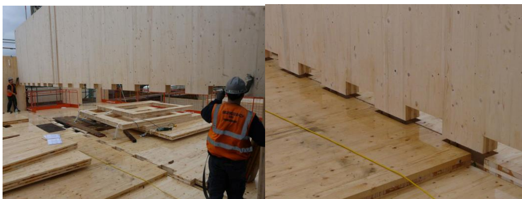
Figure 5.9: Connection of CLT wall panels to the structural timber floor at Bridport House using tongue and groove method which are properly fixed using metal base positioned at angles and screws. (Willmott Dixon, 2011)
