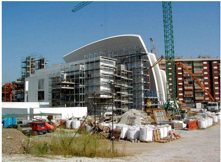
Figure 5. The northern façade of the parish house during its construction. The shells are completed and the traveling-crane disassembled (Picture by the author, taken 26/06/2012).
