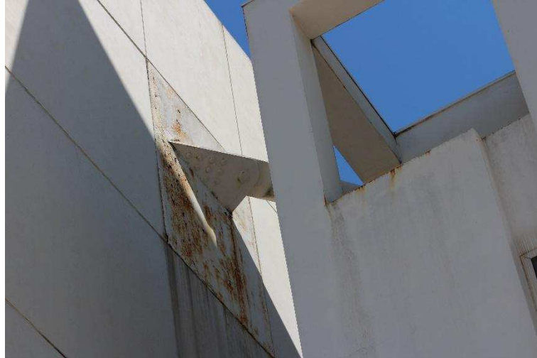
5 6 7 8 9 10 11 12 13 14 15 16 17 18 19 20 21 22 23 Figure 15. Presence of rust on the pinned joint of the roof beam (Picture by the author, taken 22/05/2016).
