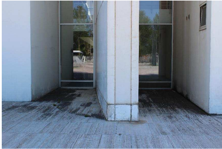
Figure 7. The area of the external pavement most affected by the acid rain deposits (Picture by the author, taken 22/05/2016).
