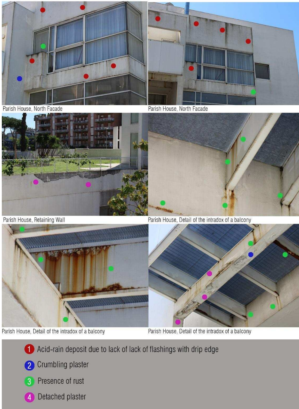
Figure 19. State of decay of the northern façade of the parish house truss (Picture by the author, taken 22/05/2016).
