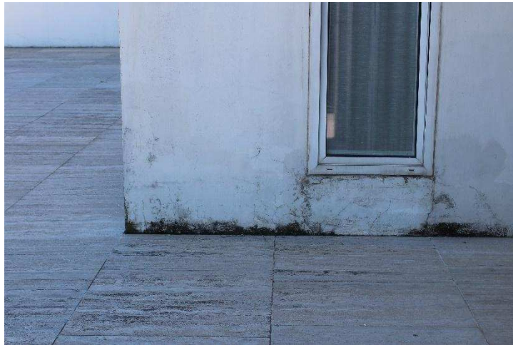
Figure 18. Mold growth at the bottom of the block of the altar.
