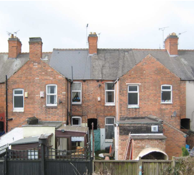
Figure 3: Terraced housing, which is superficially easy to renovate and insulate is, in the detail, surprisingly complex, especially at the rear.
