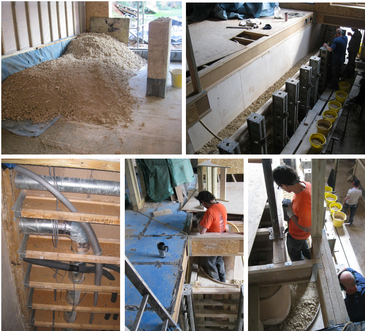
Figure 7: Top left, chalk wall testing. Top right, formwork with chalk being rammed. Bottom left: MVHR ducting crossing I-joists. Bottom right two pictures: Man ramming chalk.
