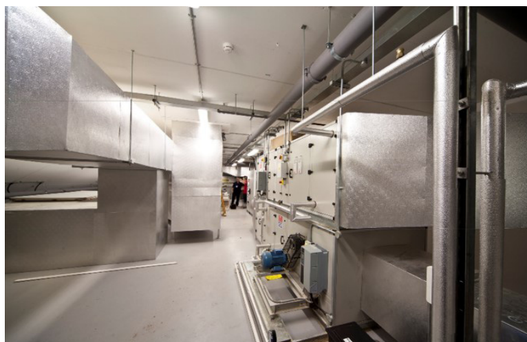
Figure 11: Interior photograph of the plant room - where all the mechanical ventilation and services are kept.
