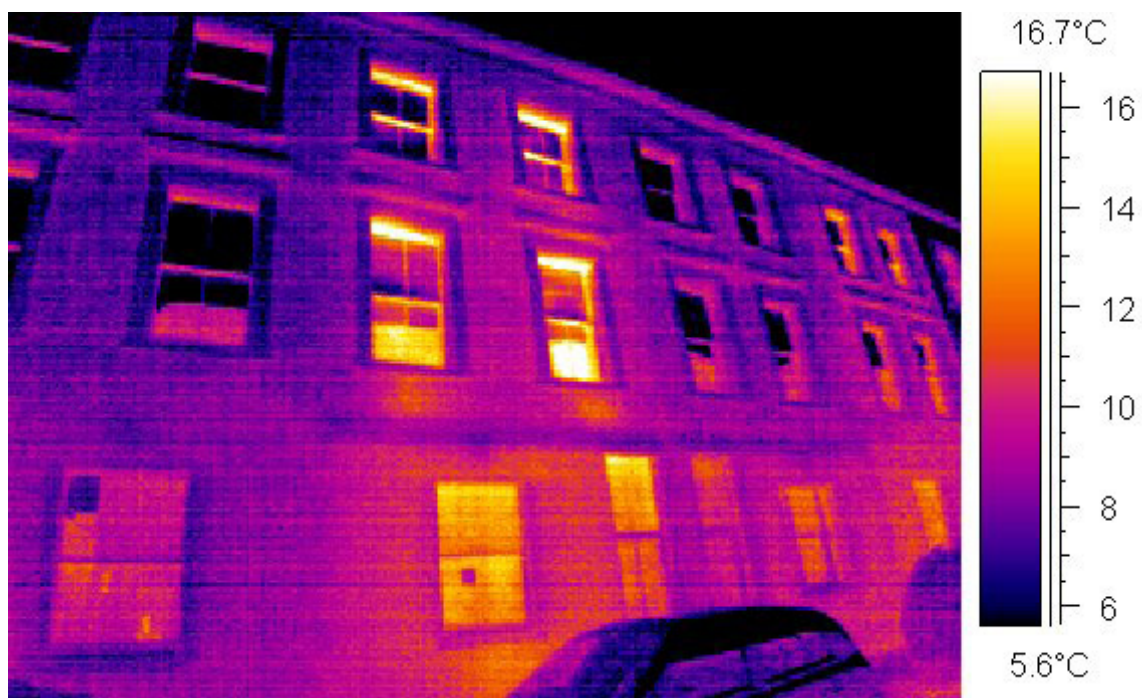
Figure 19 : A thermal imaging photograph of 100 Princedale Road as existing, showing the heat loss issues with the fabric
