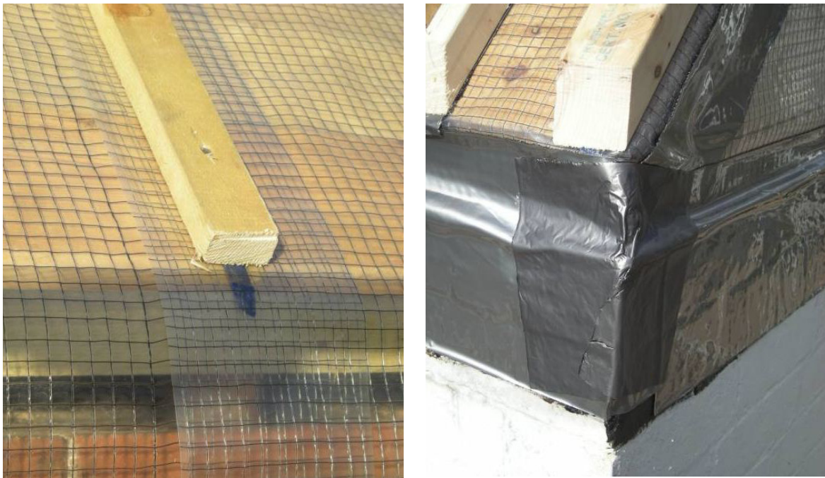
Figure 14: Airtightness membrane clamped to roof structure and sealed with bitumen tape (EST, 2010)
