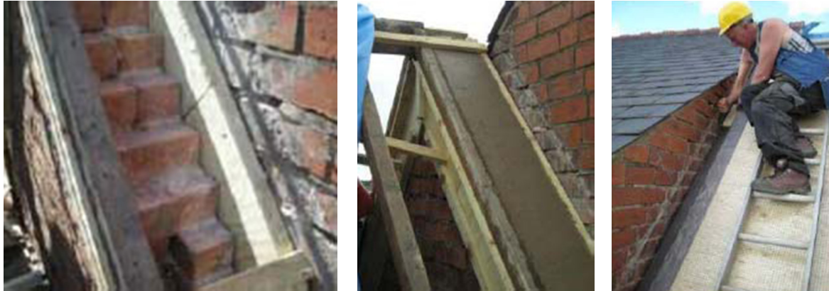
Figure 13: Repairing and making airtight the gable wall end next to the neighbouring house (EST, 2010)
