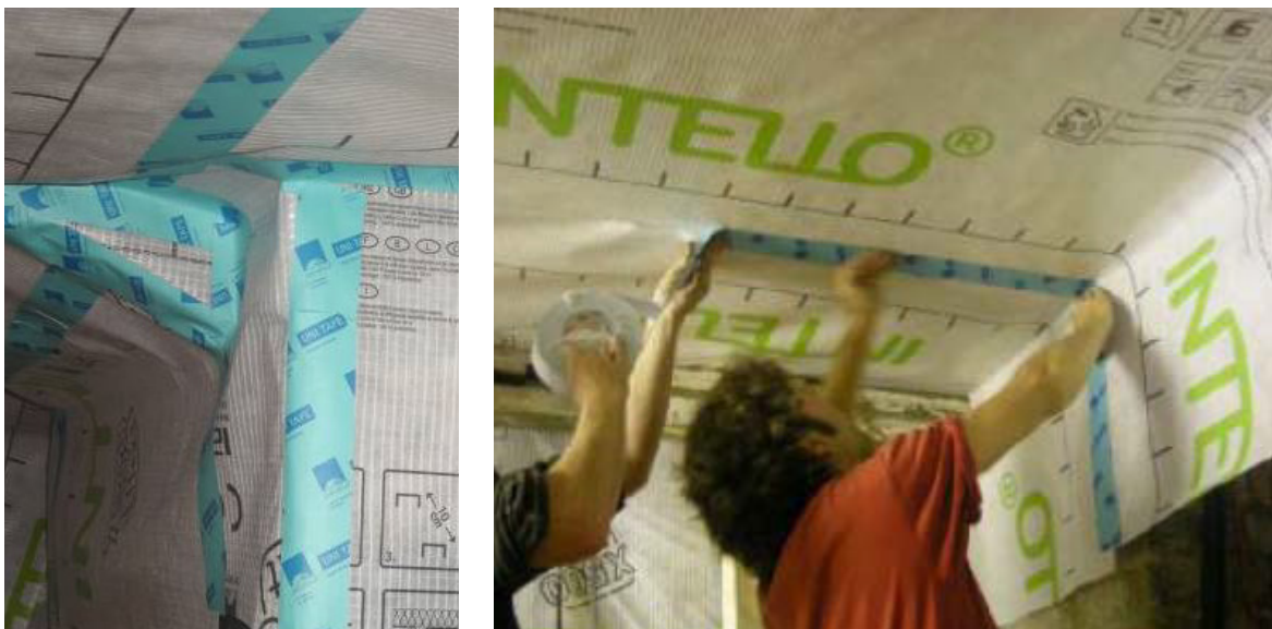
Figure 16: Applying and sealing the Intello vapour membrane to the underside of the suspended floor (EST, 2010)
