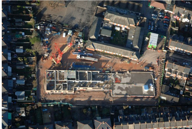
Figure 9: Photograph showing construction of the new school, it is clear to see how the concrete panels start to show the building form.
