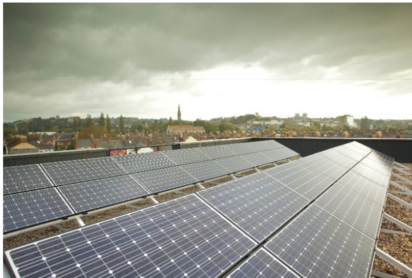
Figure 5: Photograph showing PV roof mounted panels
