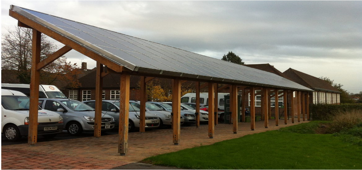
Figure 01 : Centre of Disability Studies - The entrance pergola with PV panels installation.
