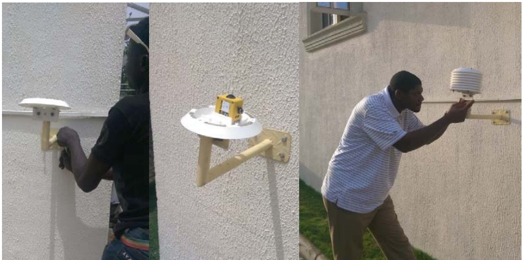
Figure 3.6: Tinytag data logger's outdoor installation with radiation shield.
