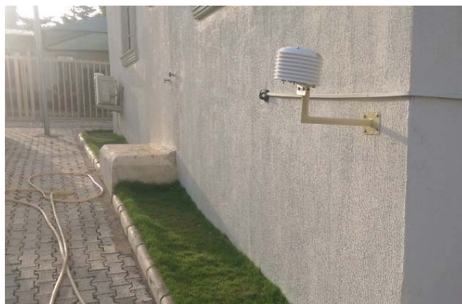
Figure 3.7: Installed Tiny Tag T/RH outdoor logger in radiation shield
