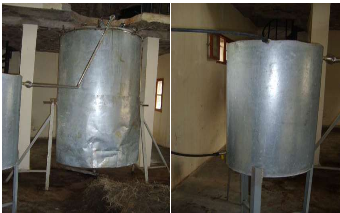
Plate 9.12: (a) The installed alembic with a capacity for 300 kilograms of plant material; (b) the condenser (El Maghzen, 2011).
