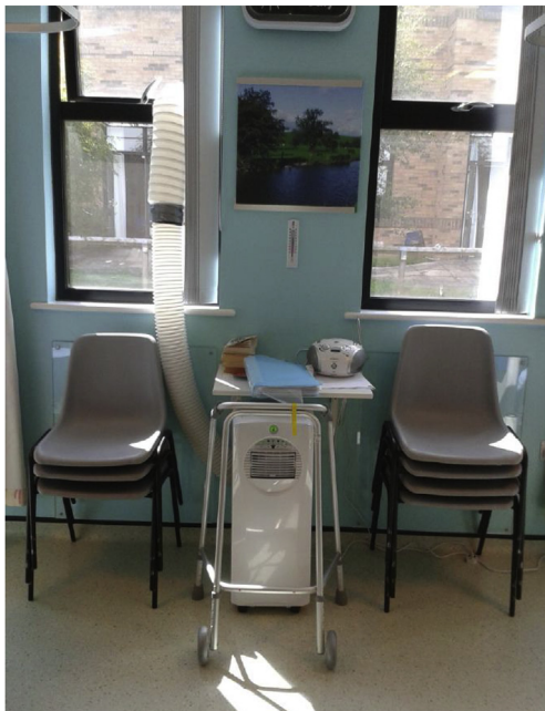
Fig. 21. Portable air conditioning unit, with makeshift safety barriers in a multi-bed room MB2 of Ward 30 during the summer of 2013.
