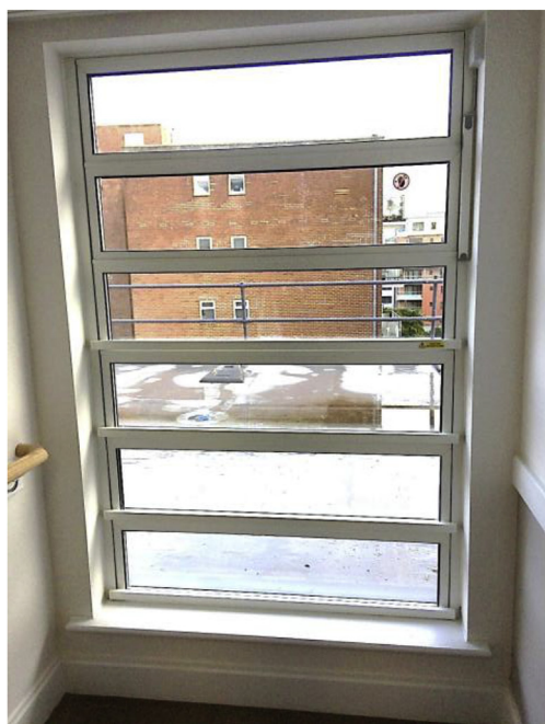
Fig. 22. A secure, safe, well-insulating window ventilation system located at the end of an otherwise blind corridor.
