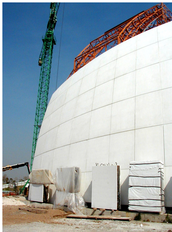
Fig. 4 The smaller shell after its completion. At its bottom some ashlar ready to be assembled for the medium-size shell. (Picture by the author, taken 04/04/2001).
