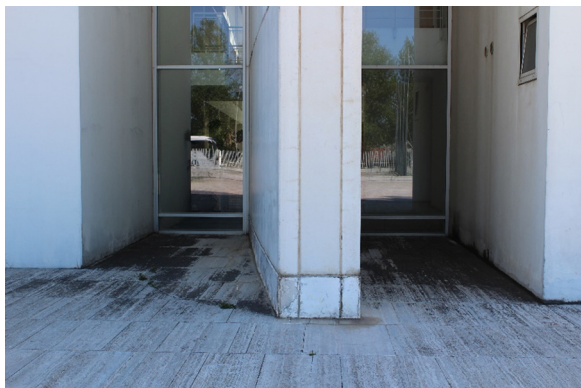
Fig. 7 The area of the external pavement most affected by the acid rain deposits (Picture by the author, taken 22/05/2016).
