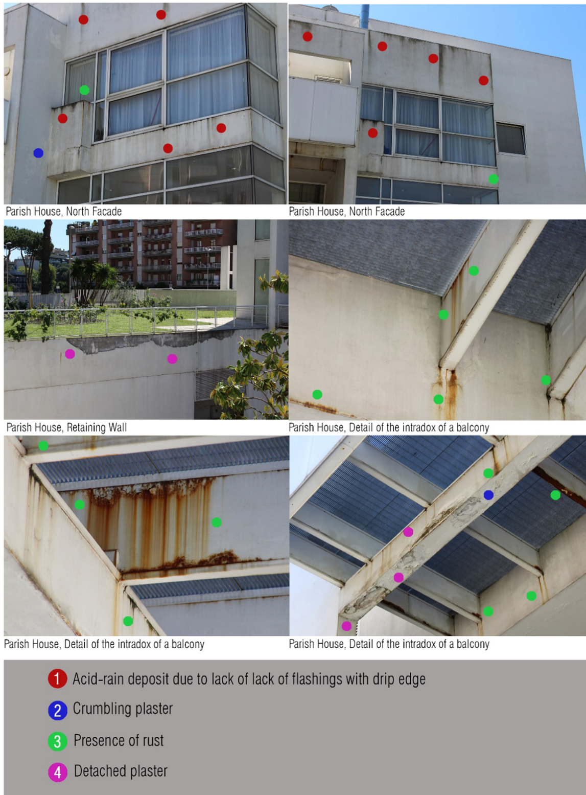
Fig. 19 State of decay of the northern façade of the parish house truss (Picture by the author, taken 22/05/2016).
