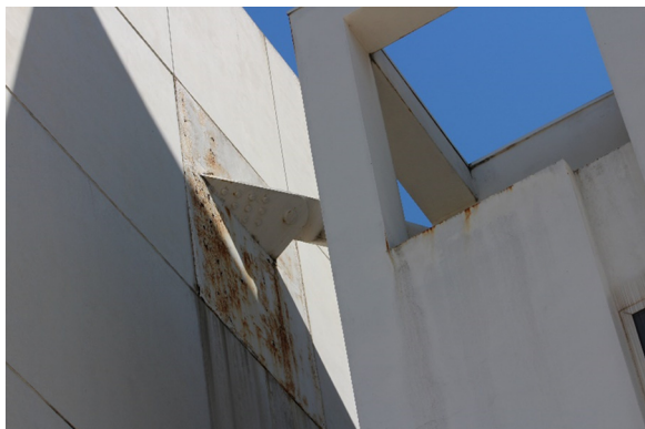
Fig. 15 Presence of rust on the pinned joint of the roof beam (Picture by the author, taken 22/05/2016).
