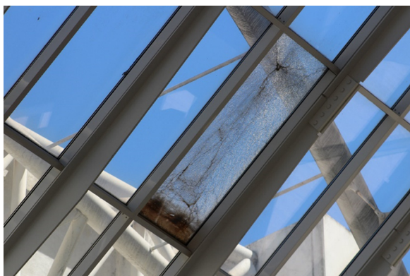
Fig. 17 A broken glass panel of the roof truss (Picture by the author, taken 22/05/2016).
