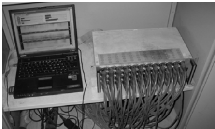
Fig.2 Flame stability monitoring system in operation
