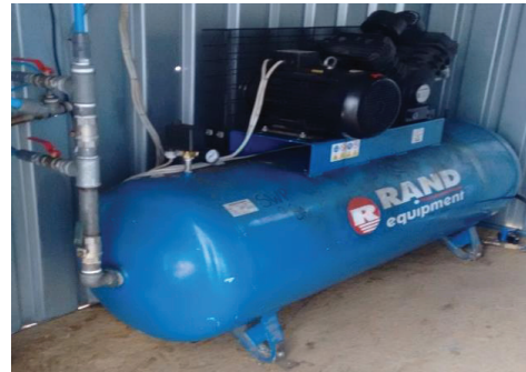
Figure 4. An air compressor system.
