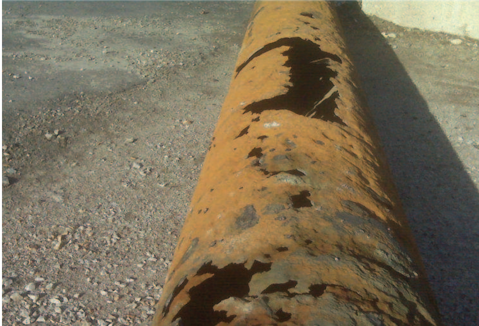
Figure 2 A new pipe in poor condition. Credit: Southern New Hampshire.
