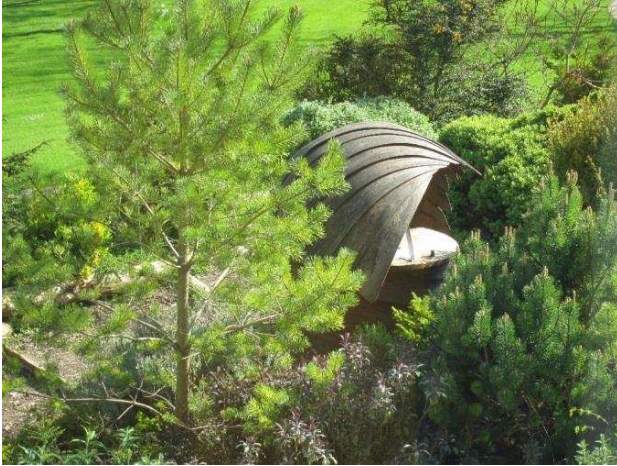
Fig 2: Cowl above inlet to earth tube
