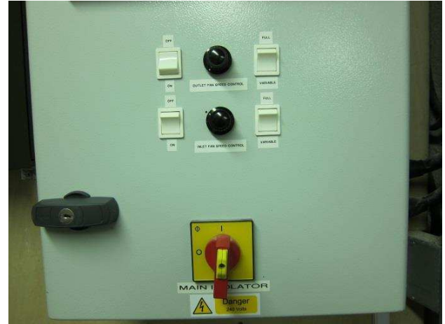
Fig 7: Fan control panel
