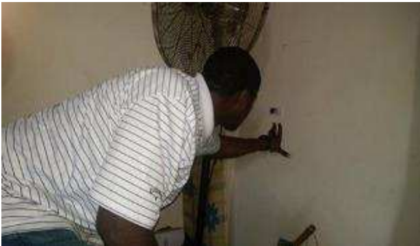
Fig 4: Installation of HOBO Temp/Rh indoor loggers
