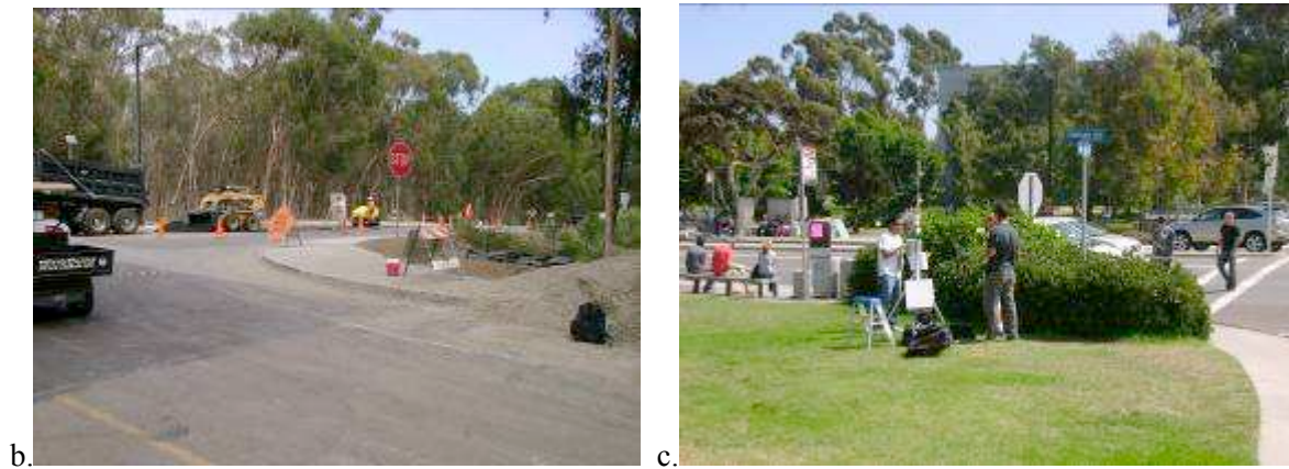
Fig. 1: (a) Overview of the survey sites (adapted from Google Earth), (b) Gilman shuttle stop TS with the DEMROES station visible in the centre, (c) Construction site CS.
