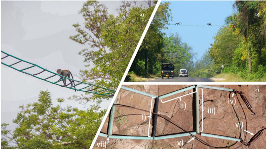
Figure 1. Horizontal ladder canopy bridges over Diani's Beach Road. a) Sykes' monkey crossing with bridge rungs visible, b) two Sykes' monkeys crossing, c) bridge components are: i) 30 cm rubber pipe, ii) 30 cm PVC conduit pipe, iii) 45 cm pressure pipe, iv) 3/16" galvanized wire rope grips, v) 3/16" galvanized wire, vi) turnbuckle.
