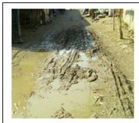
Figure 7. The area outside the Madanpur Khadar Rohingya settlement after rainfall in the month of August.
