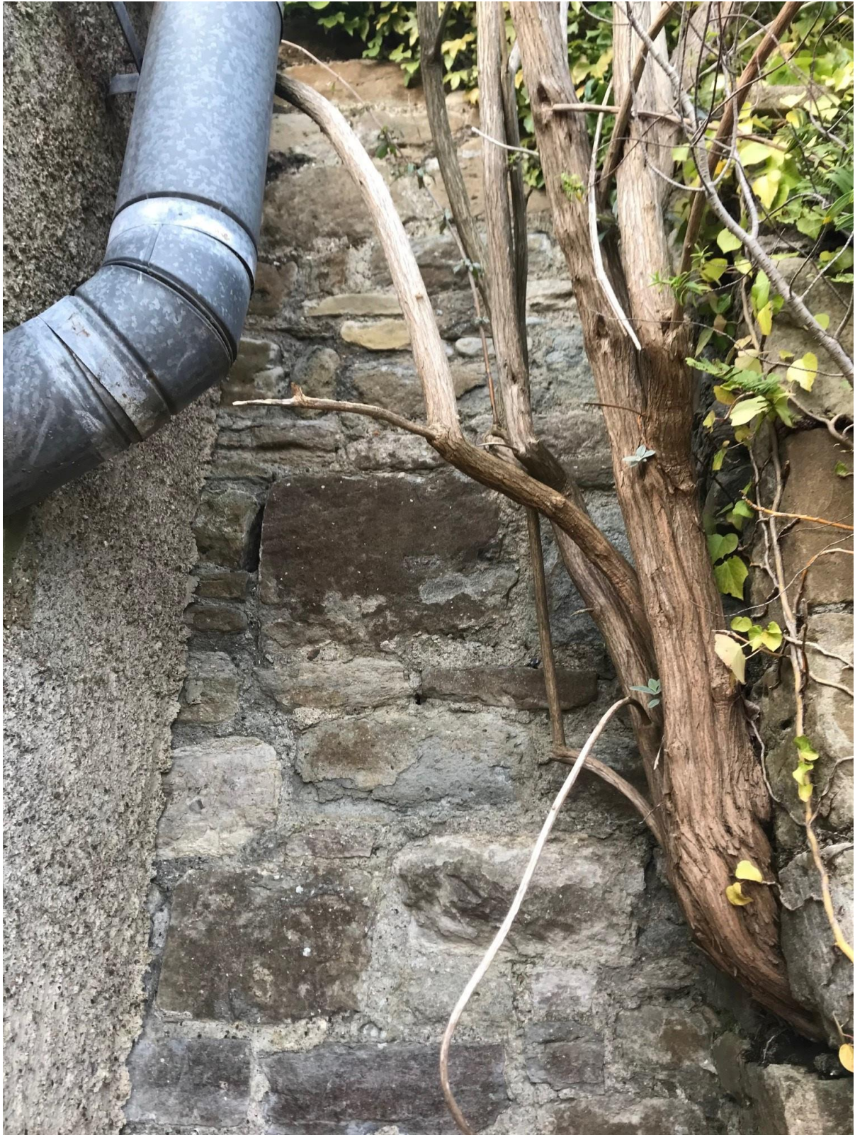
Evidence of structural failures from vegetation growth that may be used to provide substantiation for the demolition to this formerly curtilage-listed chapel
