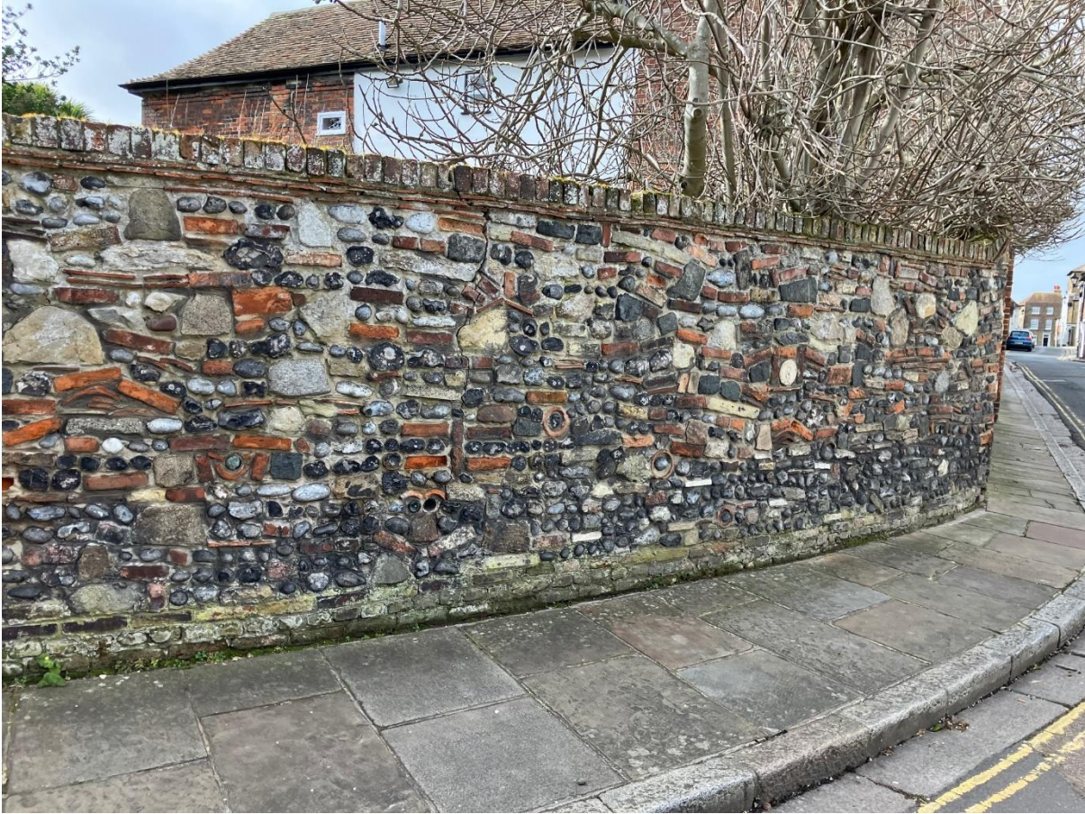
Example of spolia using stone, flint and CBM (ceramic building material) to this garden walling
