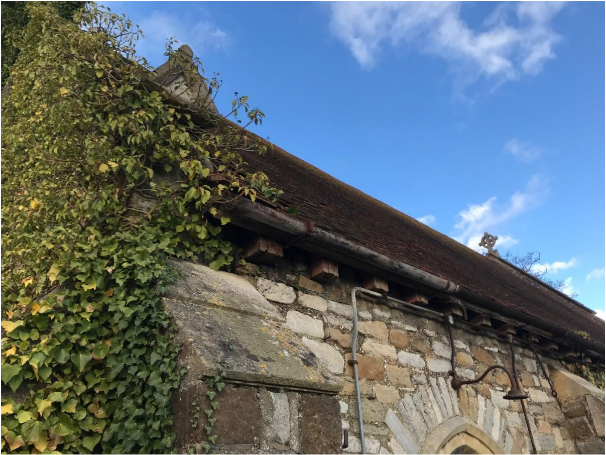
Vegetation due to no maintenance is affecting the fabric of the building
