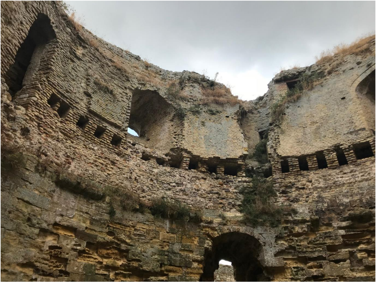
Interior of the keep showcasing a variety of latent defects
