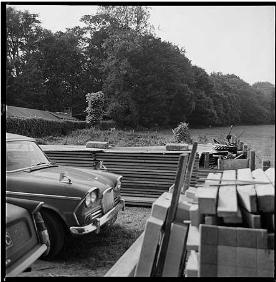
Fig. 77 Materials stored ready for use in the repair works, 1969, Historic England Archive, P/A08087/005.
