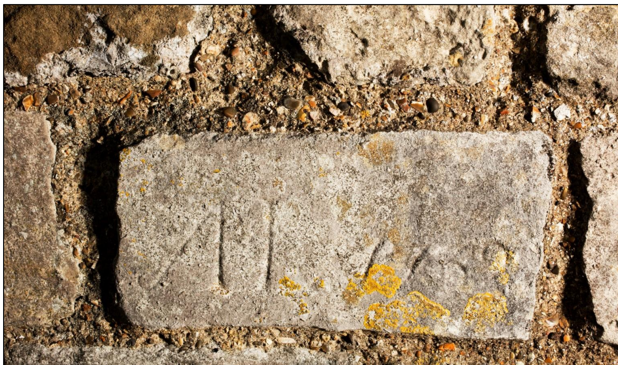
Fig. 10 Detail of the inner face of the castle's north-east inner bastion parapet, showing a stone inscribed '1732', Historic England, 2016, DP187685.
