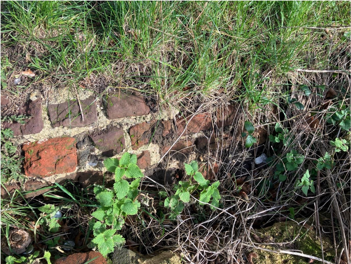
Old brickwork exposed on the Banqueting Hall as the earth around it has moved due to tree roots.
