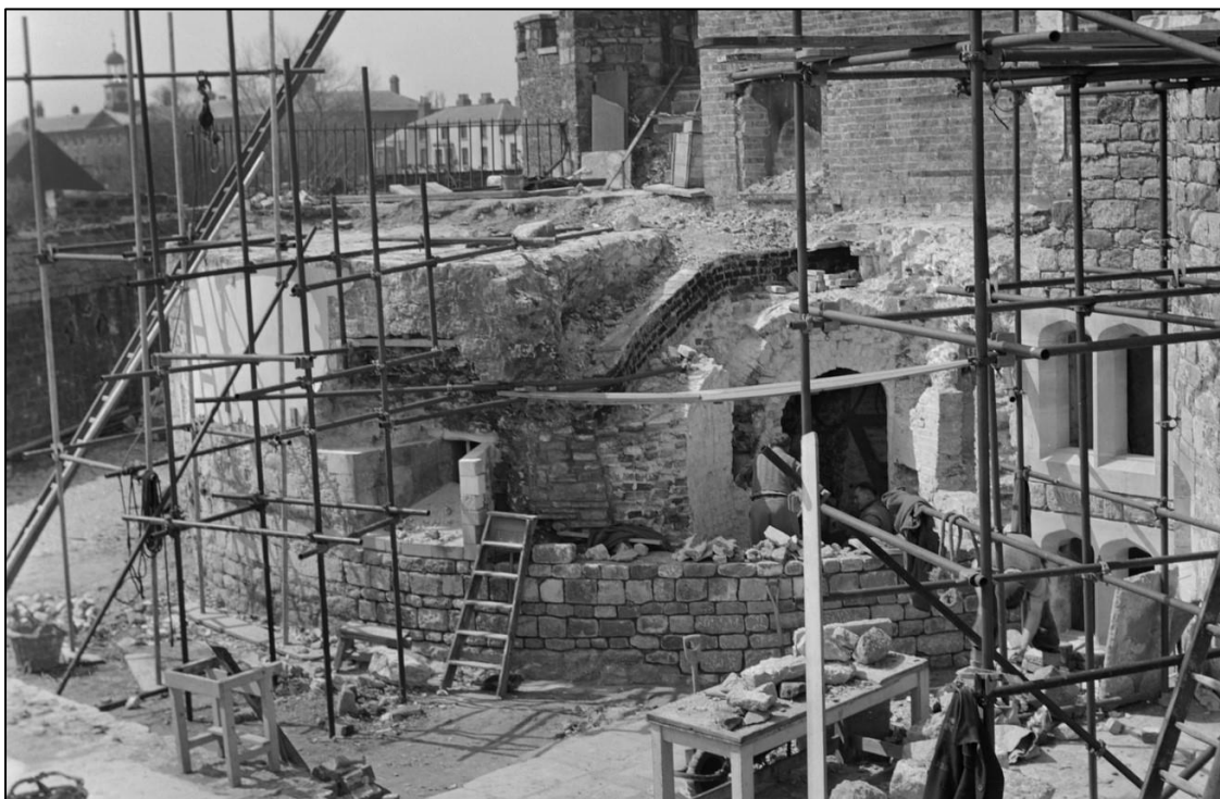
Fig. 44 Exterior view showing south-east bastion from the north-east, undergoing rebuilding, Historic England, May 1953, P/A02575/00.
