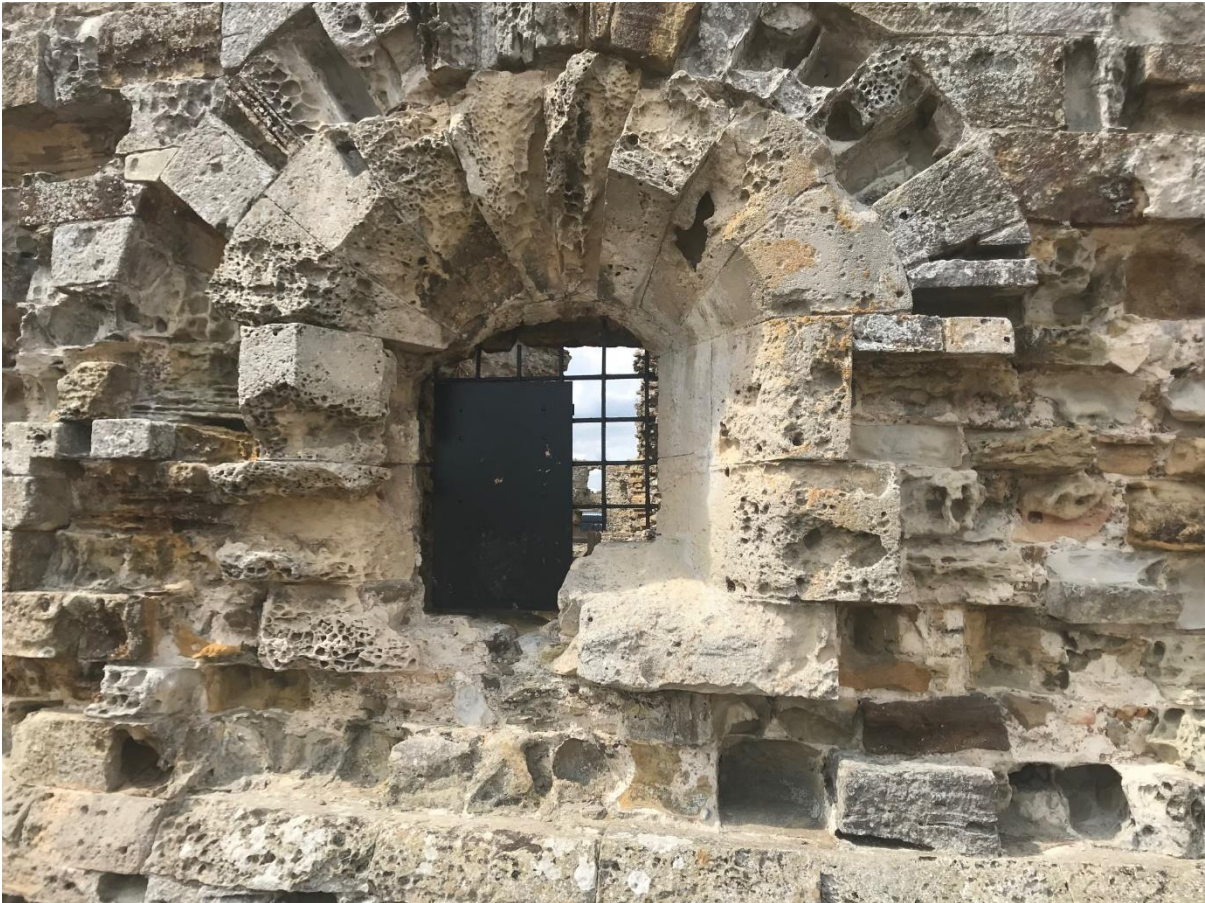
Alveolar erosion and general weathering to the outer counterscarp stonework
