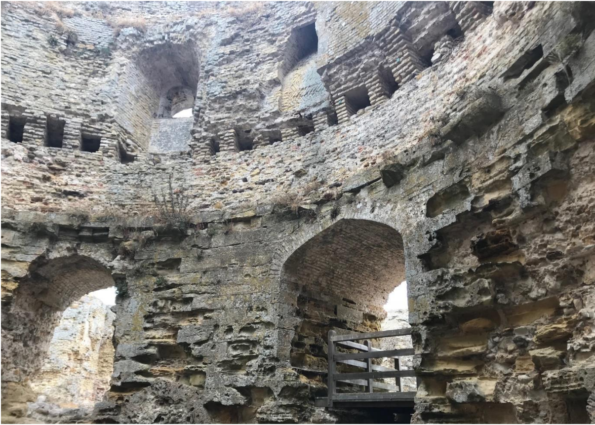
Interior of the keep showcasing a variety of latent defects
