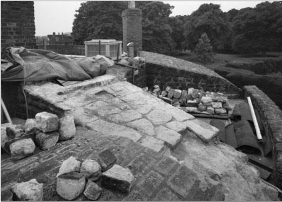
Fig. 76 Photo showing a number of stonework repairs to the coping areas of the garden-side bastion, 1966, Historic England Archives, P/A07127/004.
