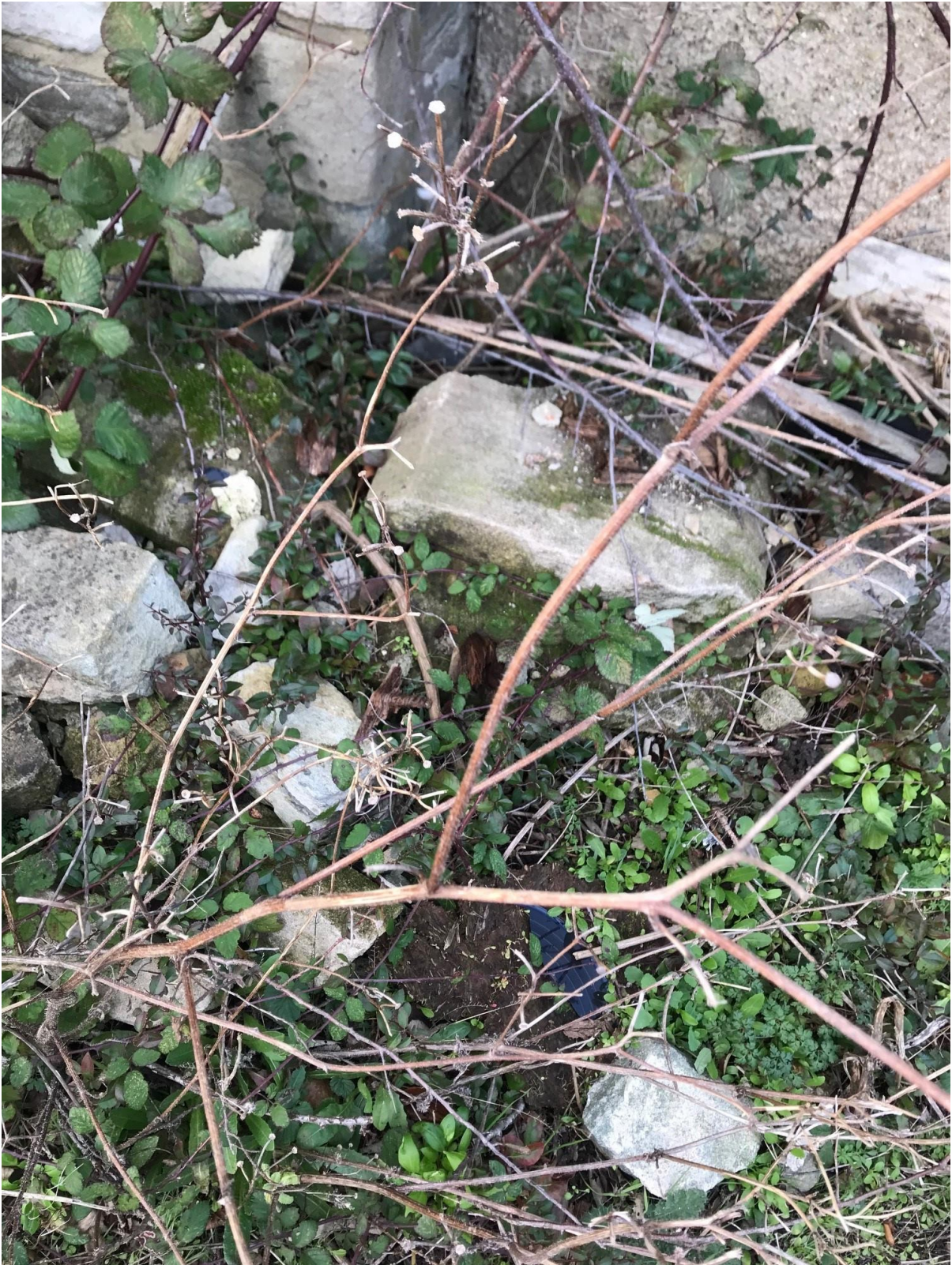
Evidence of structural failures that may be used to provide substantiation for the demolition to this formerly curtilage-listed chapel
