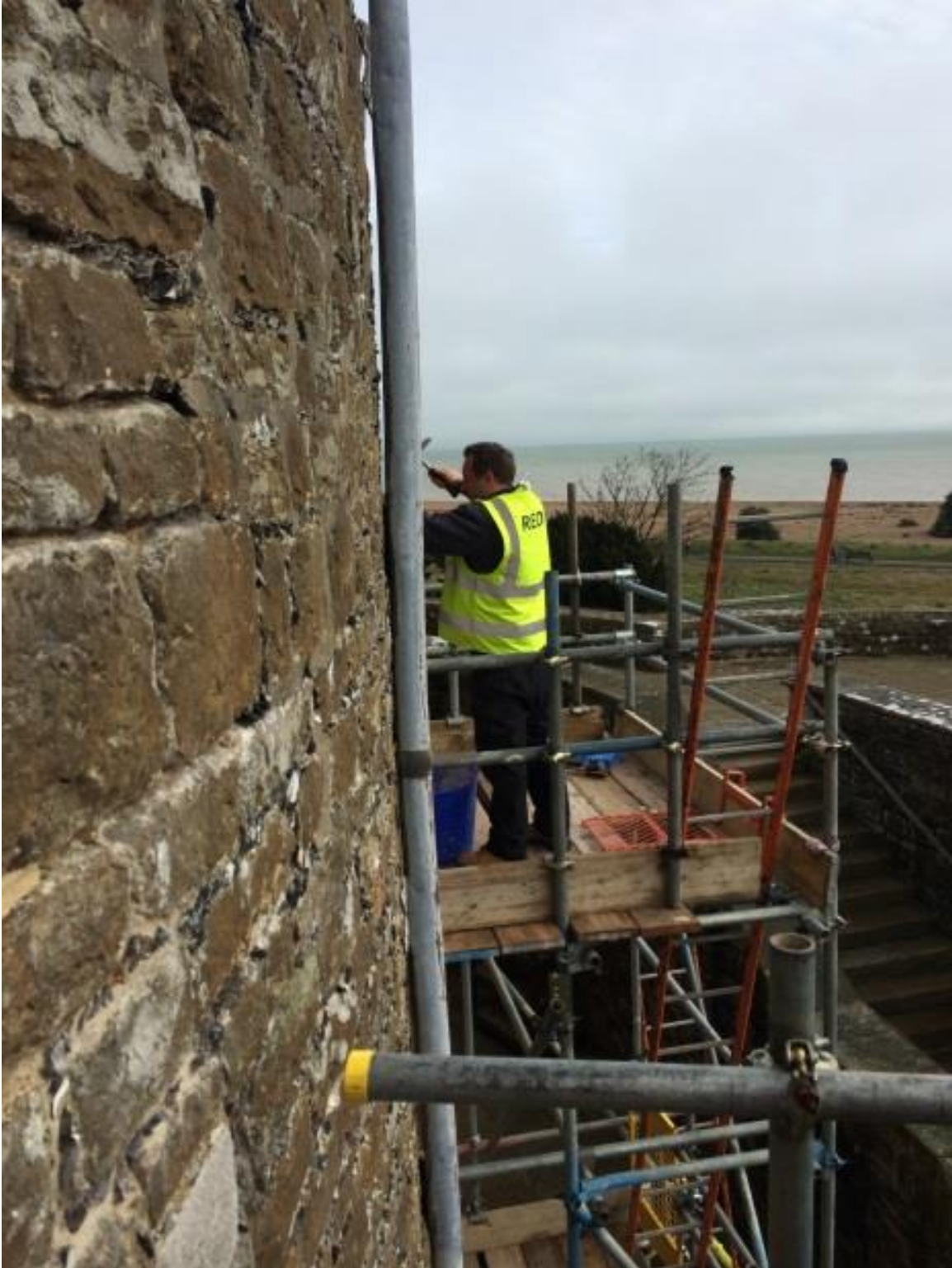
Master plasterer Gary Brisley carefully raking out cementitious mortar to the keep
