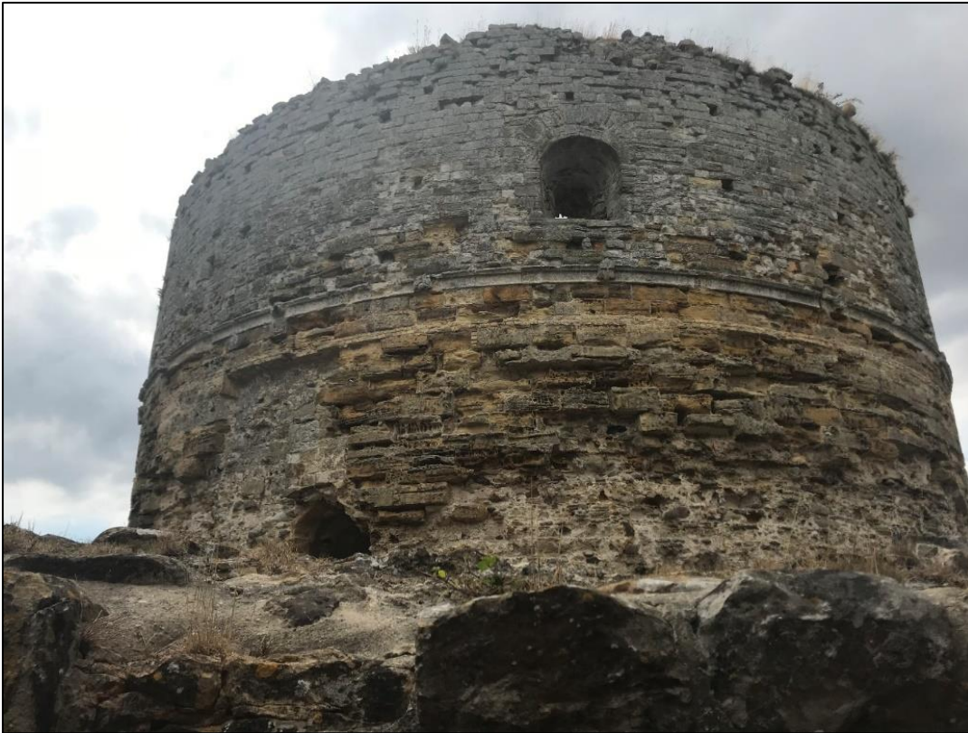
Fig. 7 Photo taken by the author of the keep at Camber Castle showing a highly worked string course and significant weathering. Site visit by the author, specially arranged with the Sussex Wildlife Trust, July 2018.
