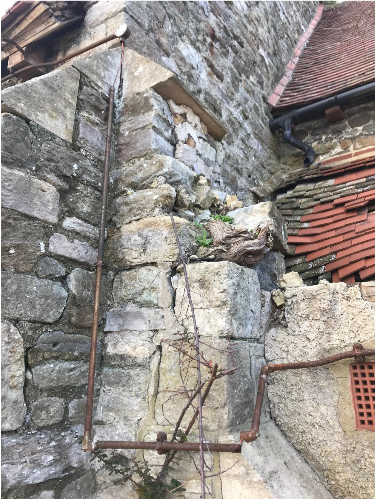
Structural collapse to the rear elevation
