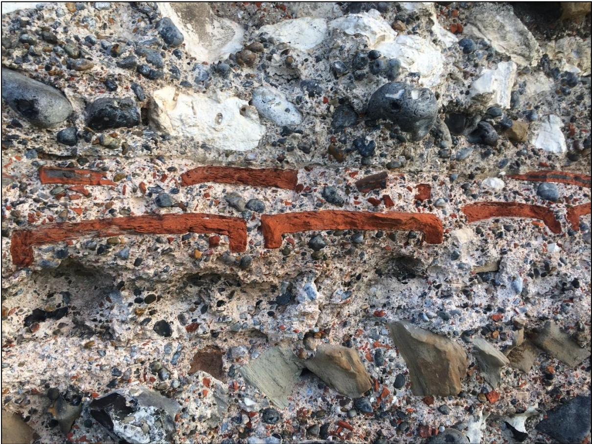
Fig. 1 A close-up of the construction of the outer walls at Richborough Castle showing Spolia use and Ceramic Building Material spolia (CBM), June 2021.
