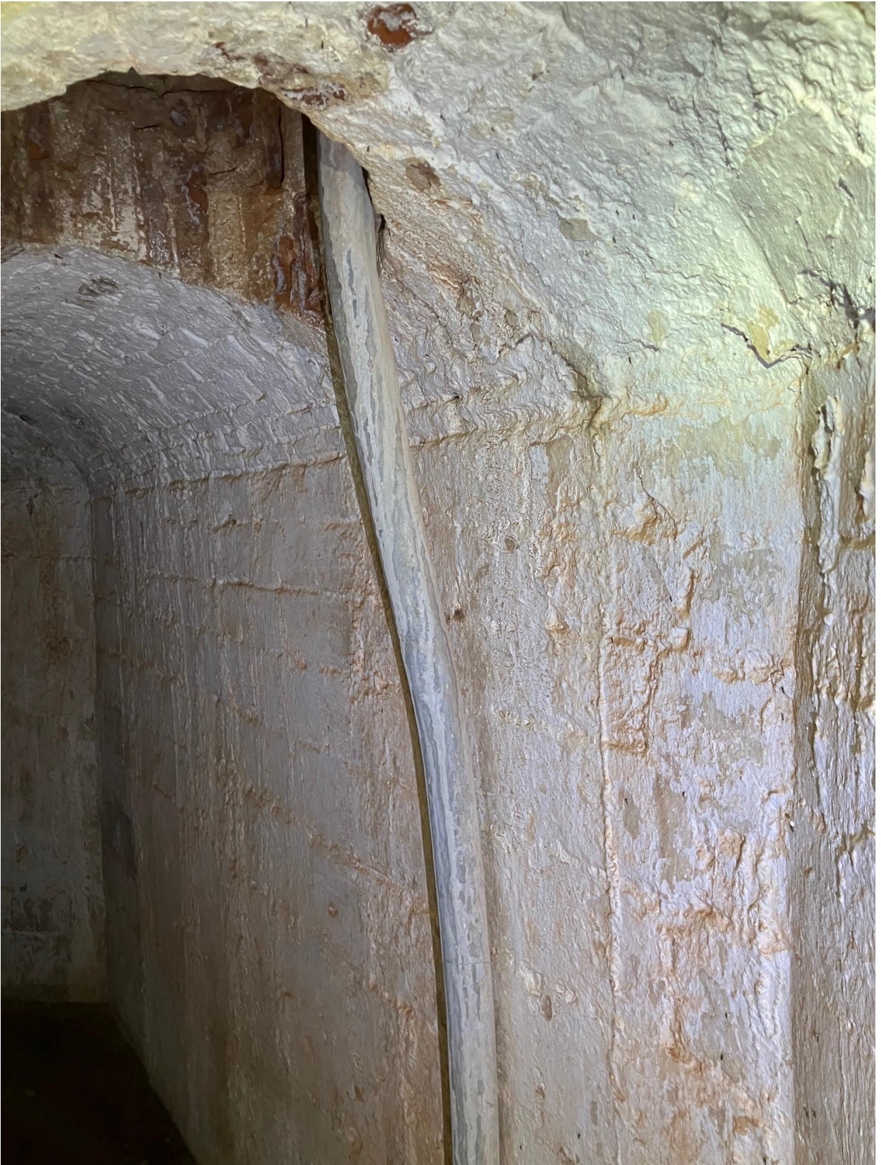
A lead downpipe, origin and termination unknown.
