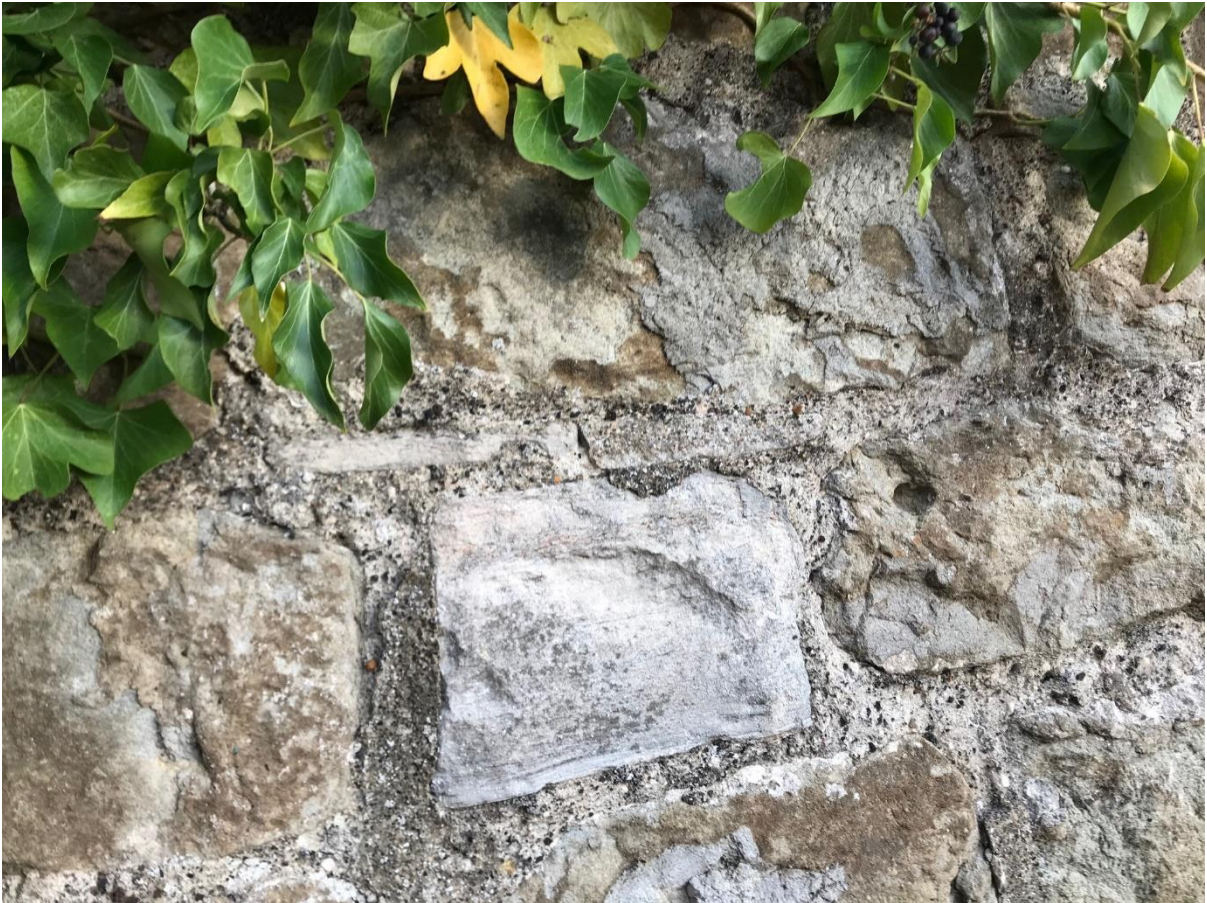
Example of spolia/medieval masonry markings in the main chapel elevations probably taken from St Radegunds Abbey via Sandown Castle
