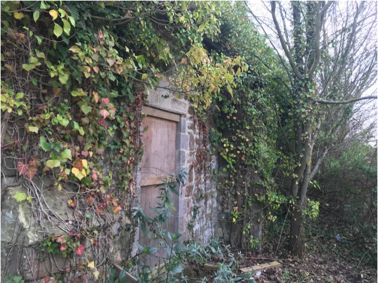
Evidence of structural failures from vegetation growth that may be used to provide substantiation for the demolition to this formerly curtilage-listed chapel
