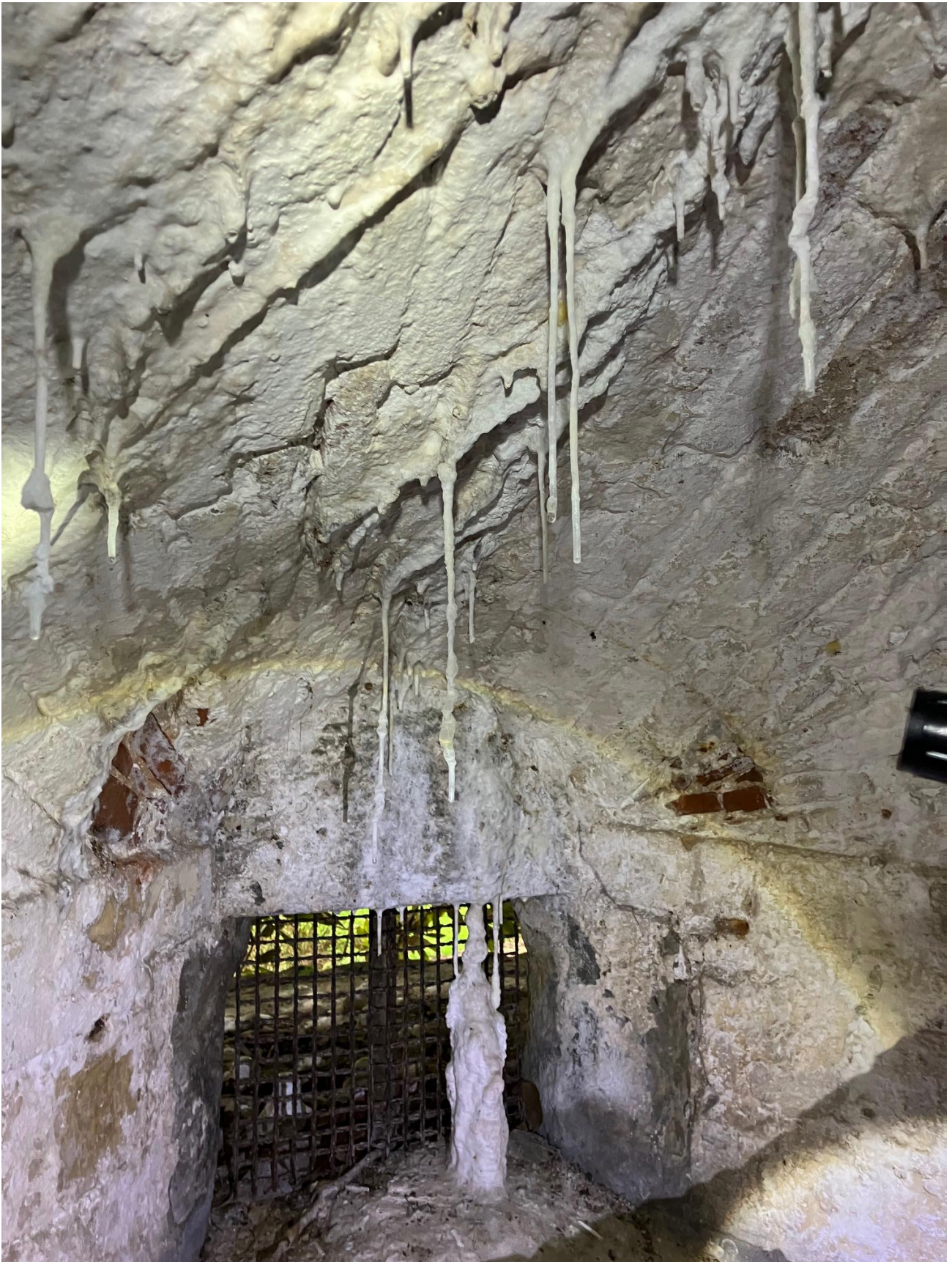
There are lots of examples of stalactites and stalagmites forming from the seaward bastions where water runs from the uncovered bastions areas and through the stonework below, depositing lime-based formations from the heavy NH lime mortar used in its construction.
