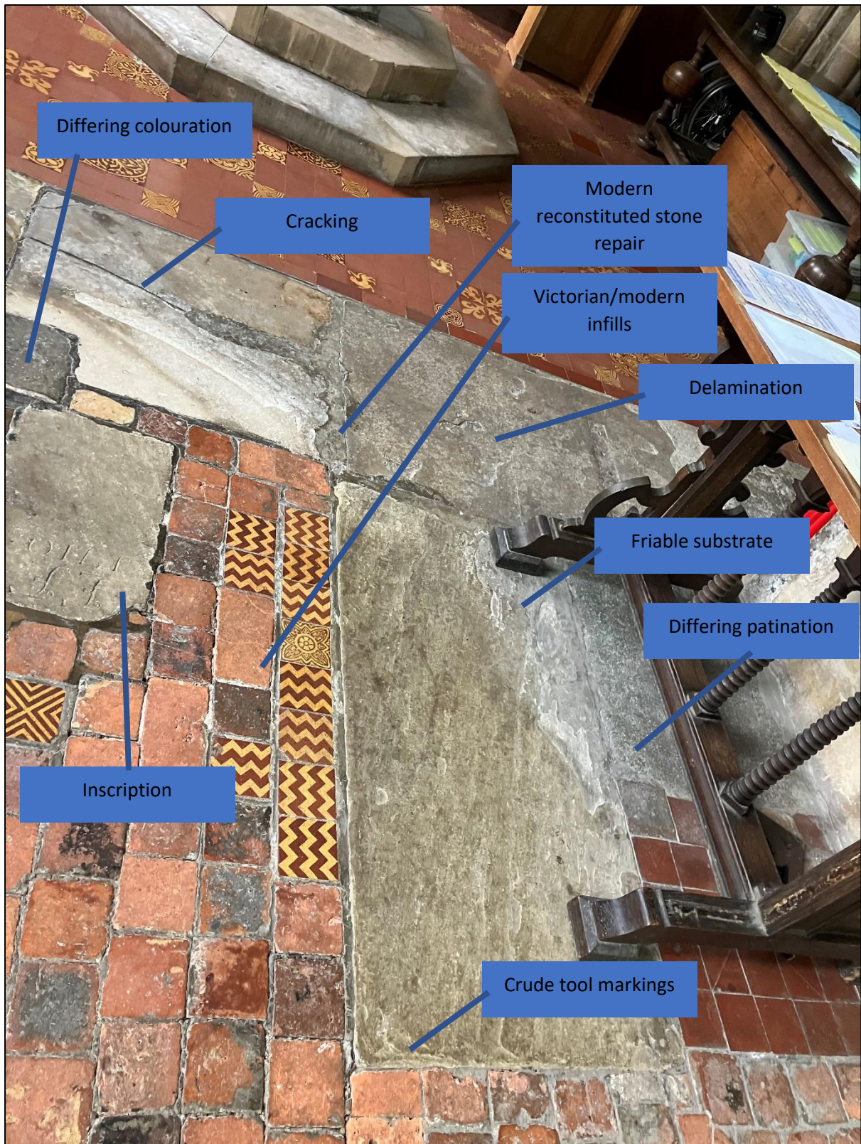
Fig. 67 Annotated photograph of the flooring in the nave of St Clement's Church Sandwich, showing the spolia Purbeck Marble floor slabs and their signs of age-related deterioration and wear, photograph by the author, 2022.
