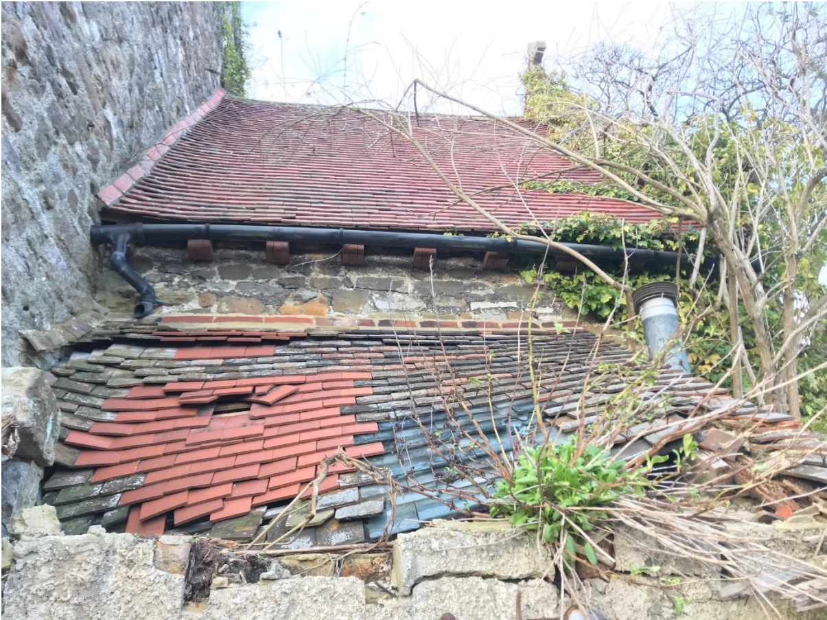
A later lean-to building (possible outhouse) is suffering from structural decline
