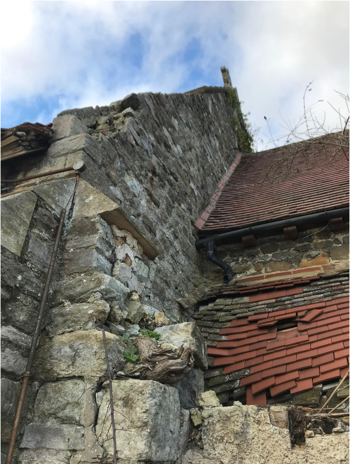
Easterly elevation buttress is collapsing from lack of maintenance. The large Kentish ragstones are evidenced with Caen stone copings – the latter is very uncommon and unique for a vernacular chapel of this location.
