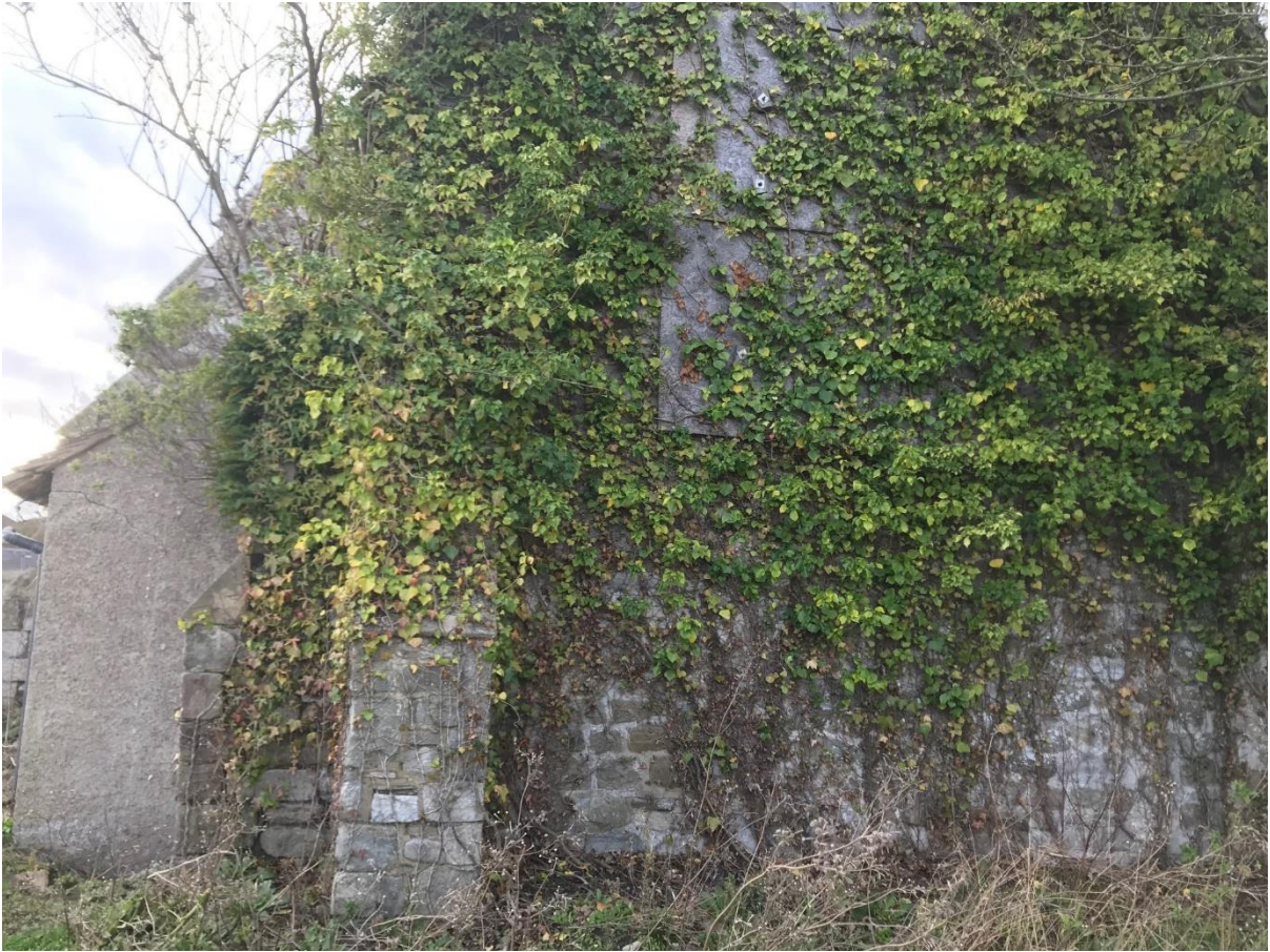
Evidence of structural failures from vegetation growth that may be used to provide substantiation for the demolition to this formerly curtilage-listed chapel
