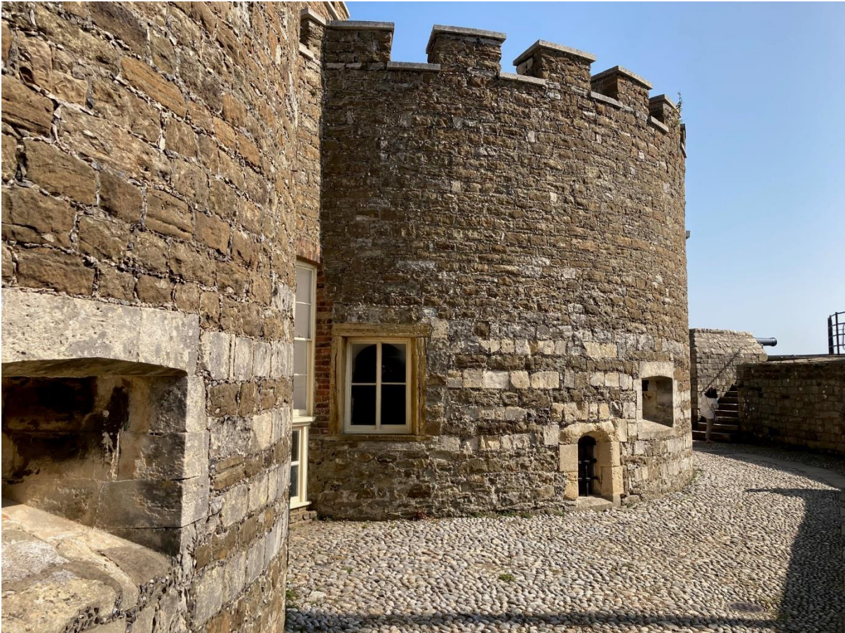
Inner bastions from the bailey showing the extent of freestone spolia as deployed by the Tudor builders
