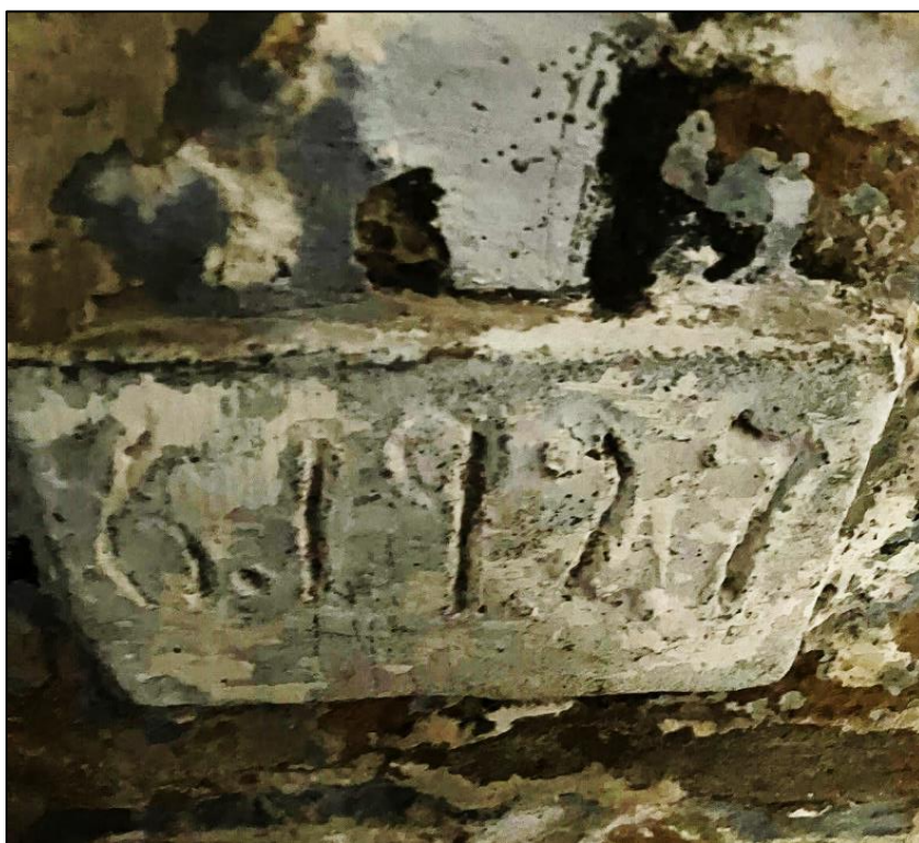
Fig. 29 A photograph by the author of the in-situ precision gauges used in 1927 to detect structural issues at the Castle. The 'six' likely denotes June and others have 'eight', likely denoting August 1927, 2023.
