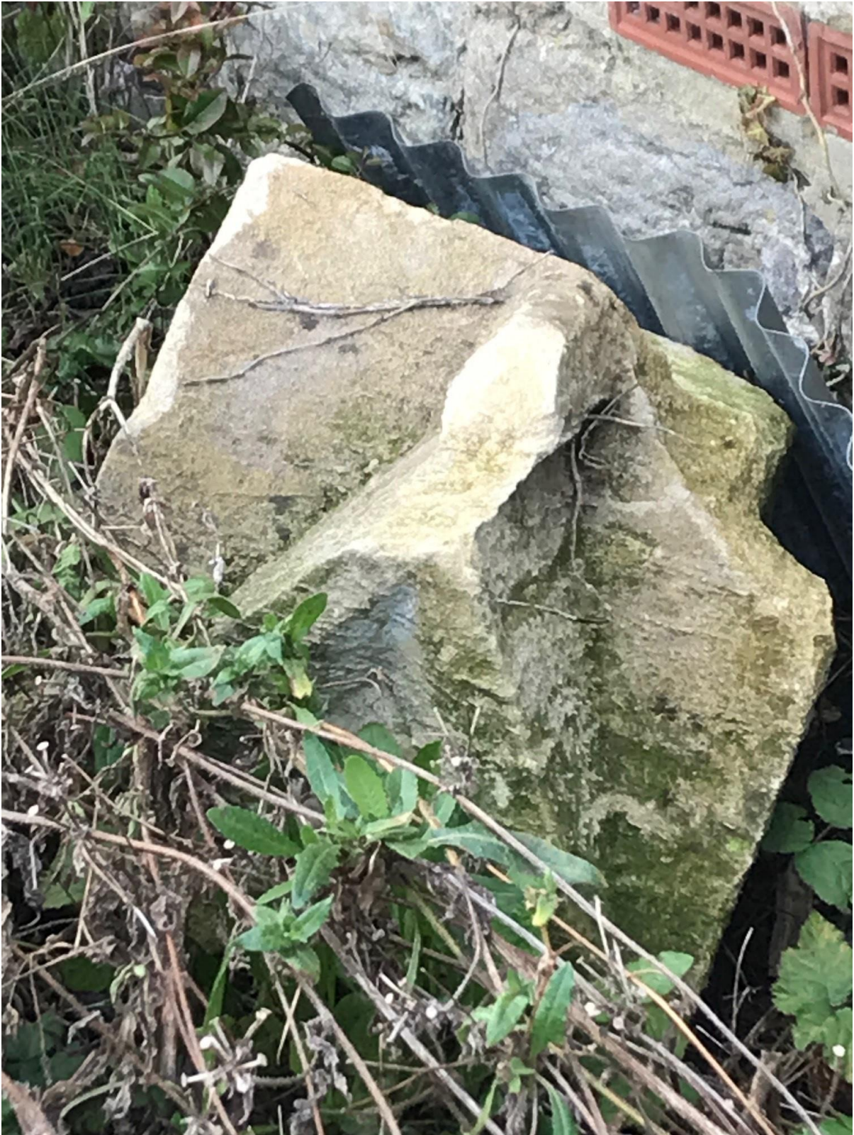
Evidence of structural failures that may be used to provide substantiation for the demolition to this formerly curtilage-listed chapel
