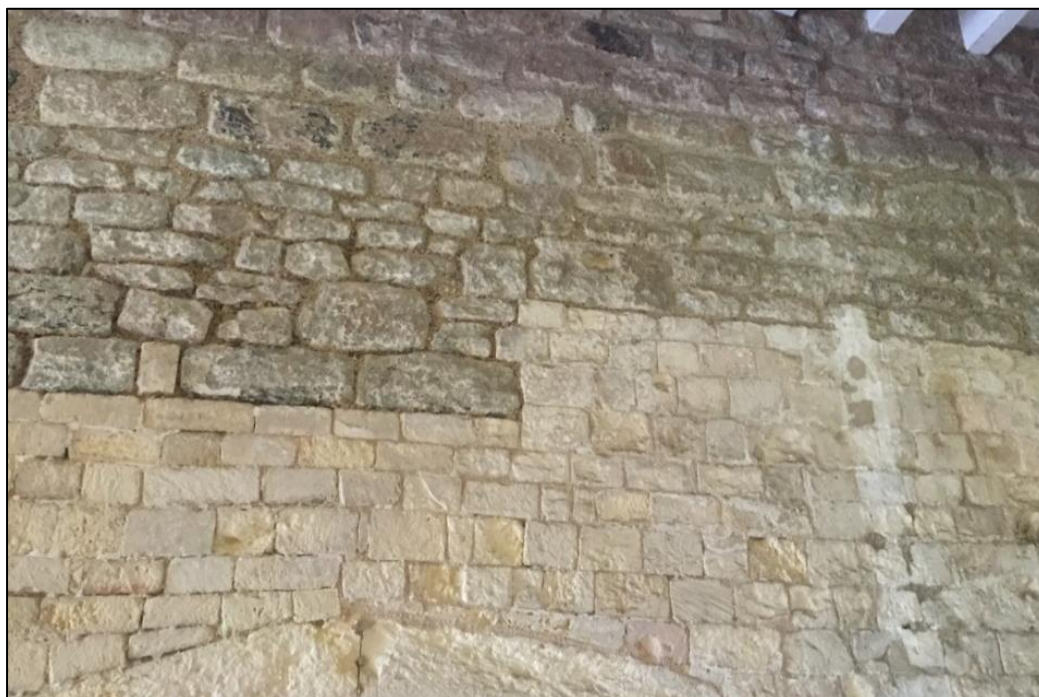
Fig. 56 Photograph of the stonework in the entrance bastion at Walmer Castle (photo author, 2019).
