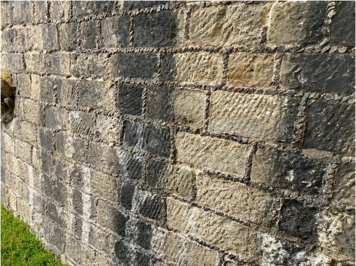
Close-up of the exterior stonework showing a well-mined, cut and prepared Kentish ragstone with galletted pointing
