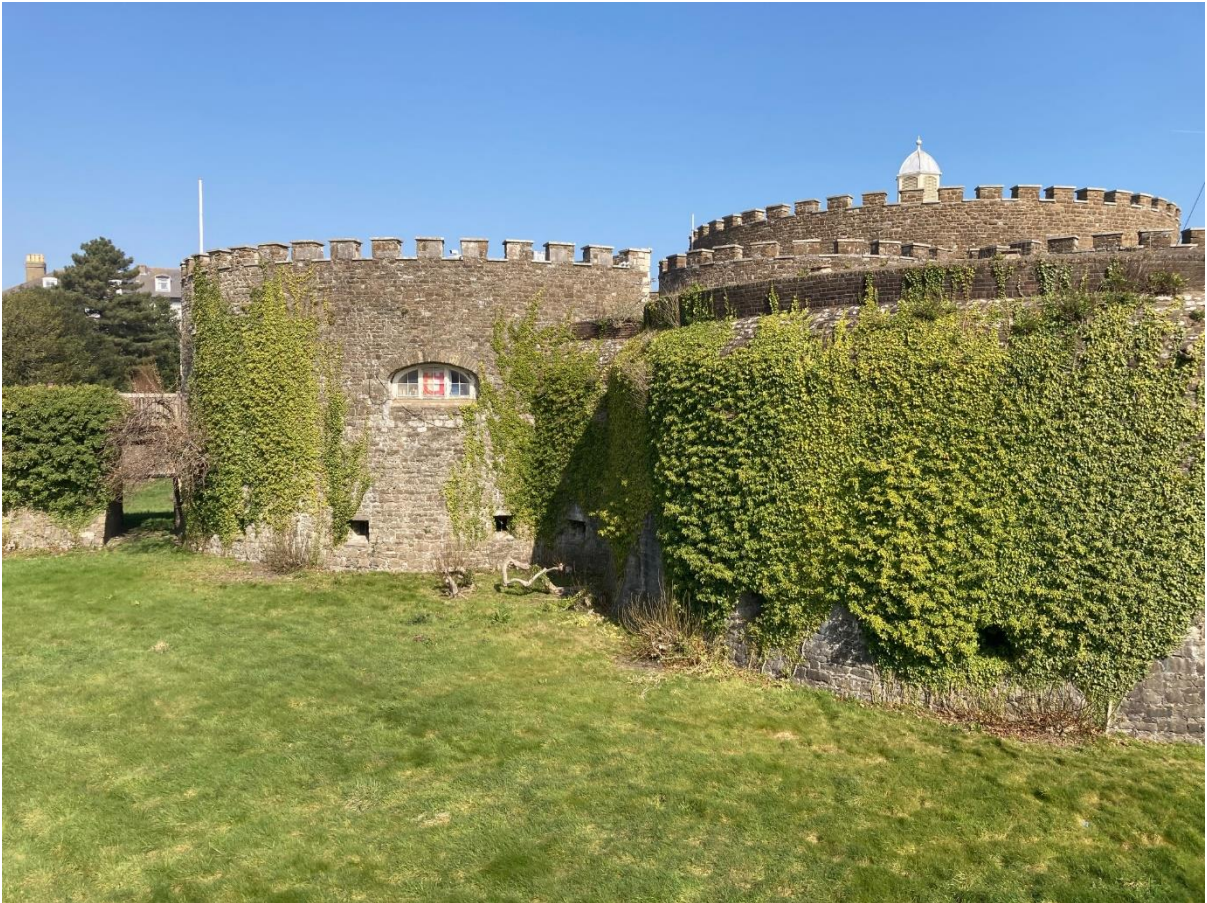
Grassed moat and vegetation growing onto the monument
