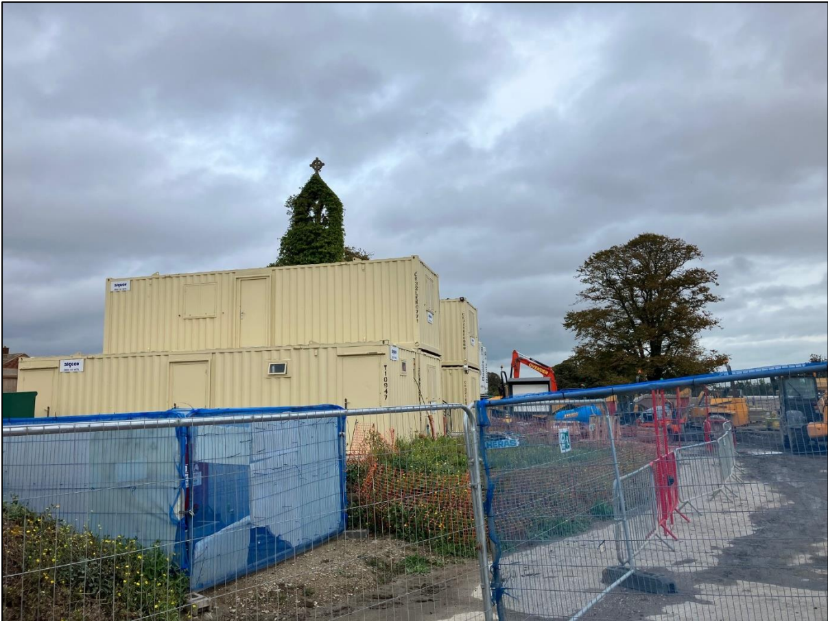
Fig. 5 The current construction site for new build housing surrounding Eastry Chapel, October 2023.
