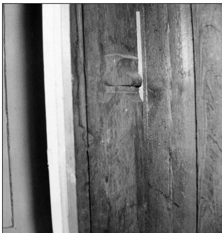
Fig. 25 Photograph from 1966 showing the original oak Tudor partitions hidden behind much-later additions, Historic England Archive, AL0960/064/04.
