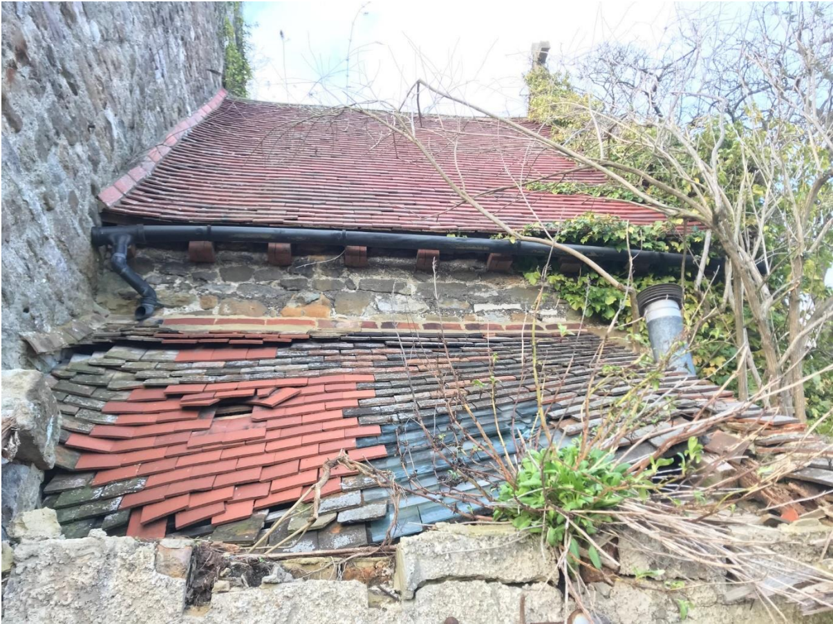
Significant water ingress and structural issues are being caused by this mid-C20th lean-to that is failing and causing damage to the interior of the chapel
