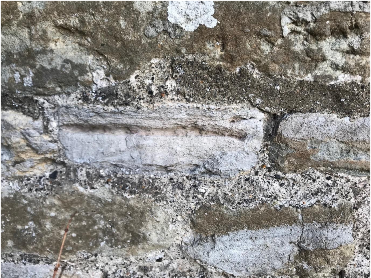
Example of spolia/medieval masonry markings in the main chapel elevations as probably taken from St Radegunds Abbey via Sandown Castle
